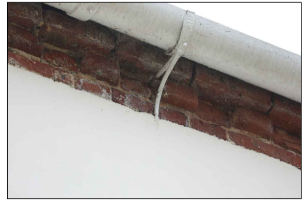
HALF ROUND CAST IRON GUTTER WITH METAL SUPPORT BRACKETS GROUTED INTO MASONRY
