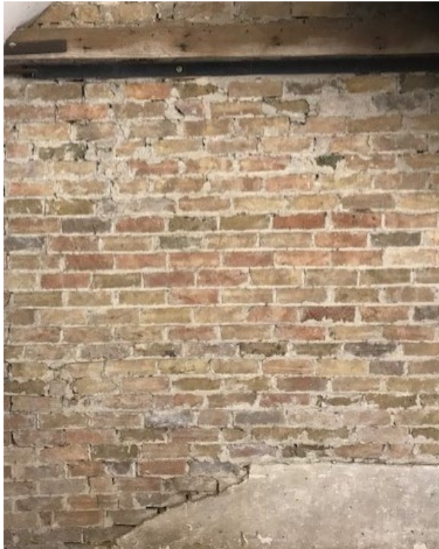
Photograph 4 - First floor single skin gault brickwork partition in which the opening to the bathroom will be created.
