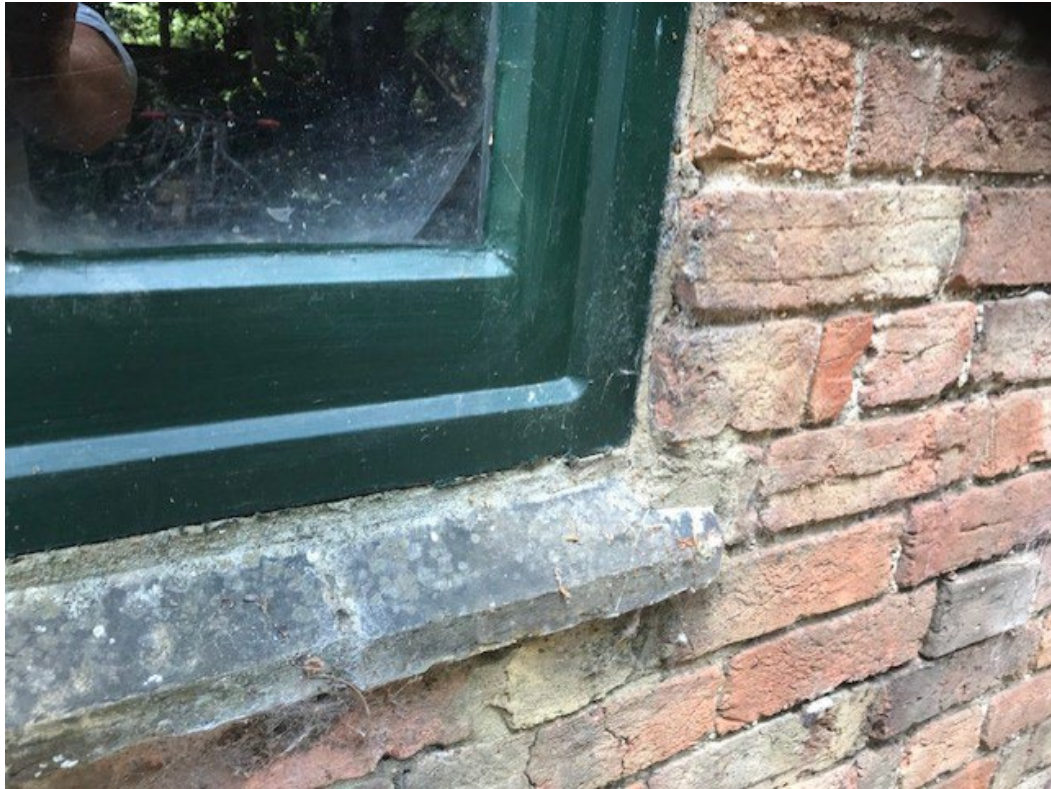
Photograph 5 - Ground floor modern, non-opening window frame flush with the brickwork to be replaced.
