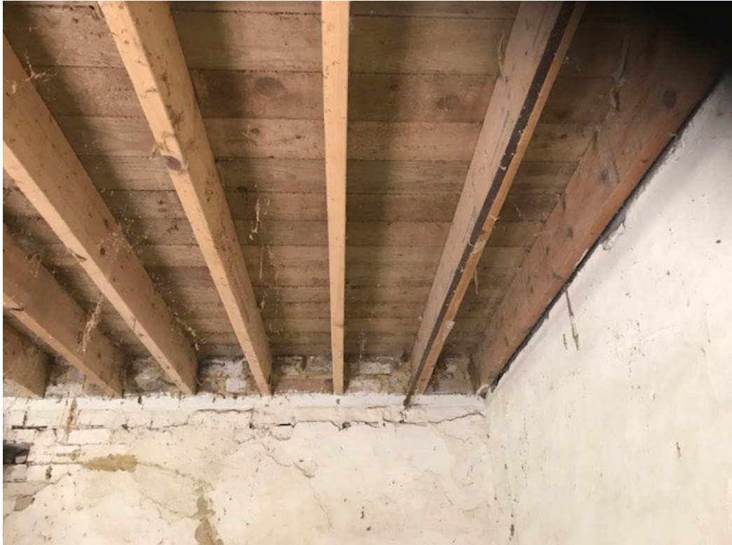
Photograph 3 - Modern timber first floor structure in which the staircase opening will be cut.
