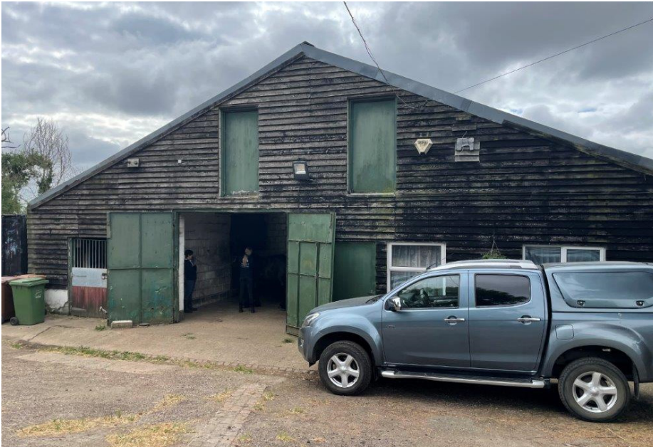
Front elevation of barn building facing Crossoaks Lane. The Flat occupies the right side.
