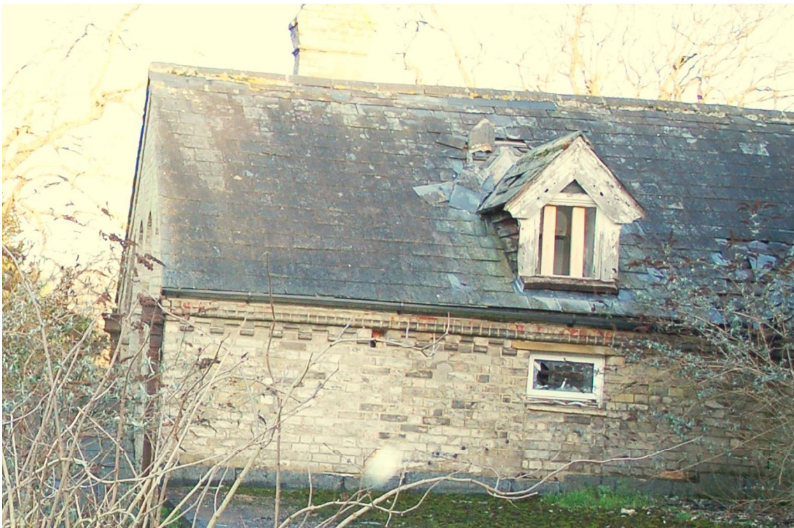
Damaged Slate Roofing
