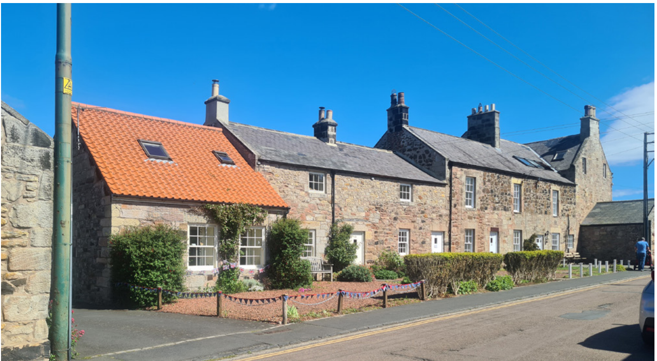
Figure 6. There are clear signs of alterations to the façades and historic fabric of 6-14 The Wynding. Interventions into the stonework are also visible.
