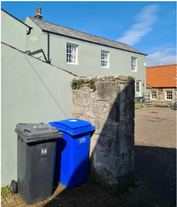
Figure 12. Existing stone wall separating 4-4A The Wynding from the rest of the properties.
