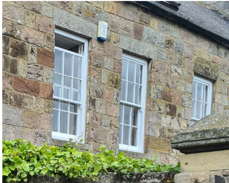
Fig 26. Unoriginal timber windows to be replaced with operational timber sash windows with double glazed conservation type units.
