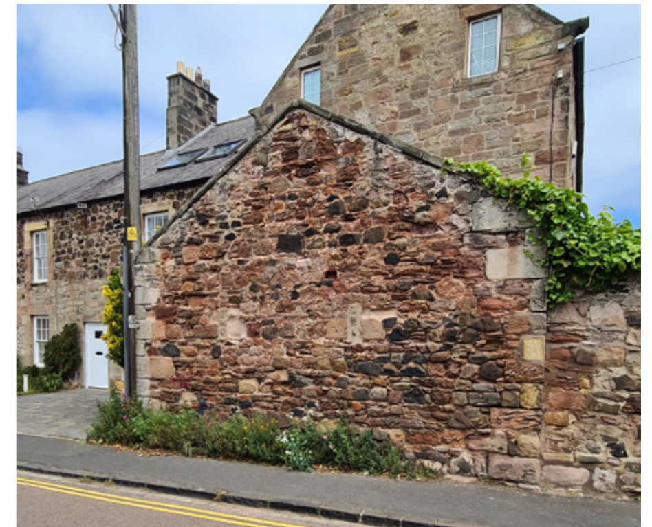
Fig 23. Significant deterioration to the rubble wall of the garage.
