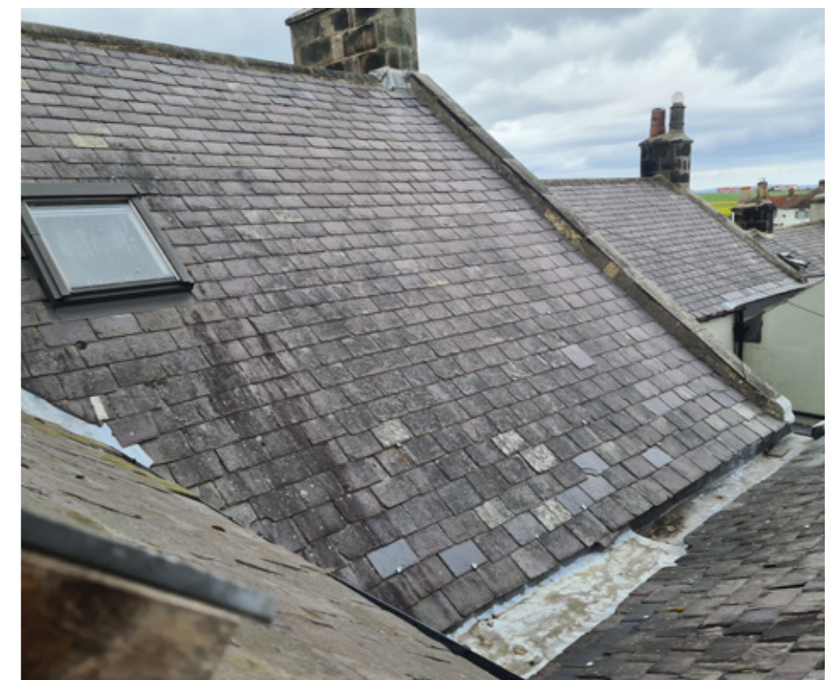
Fig 25. Proposed Welsh slate roof to be removed and replaced to match existing with aim to re-use the original slate.
