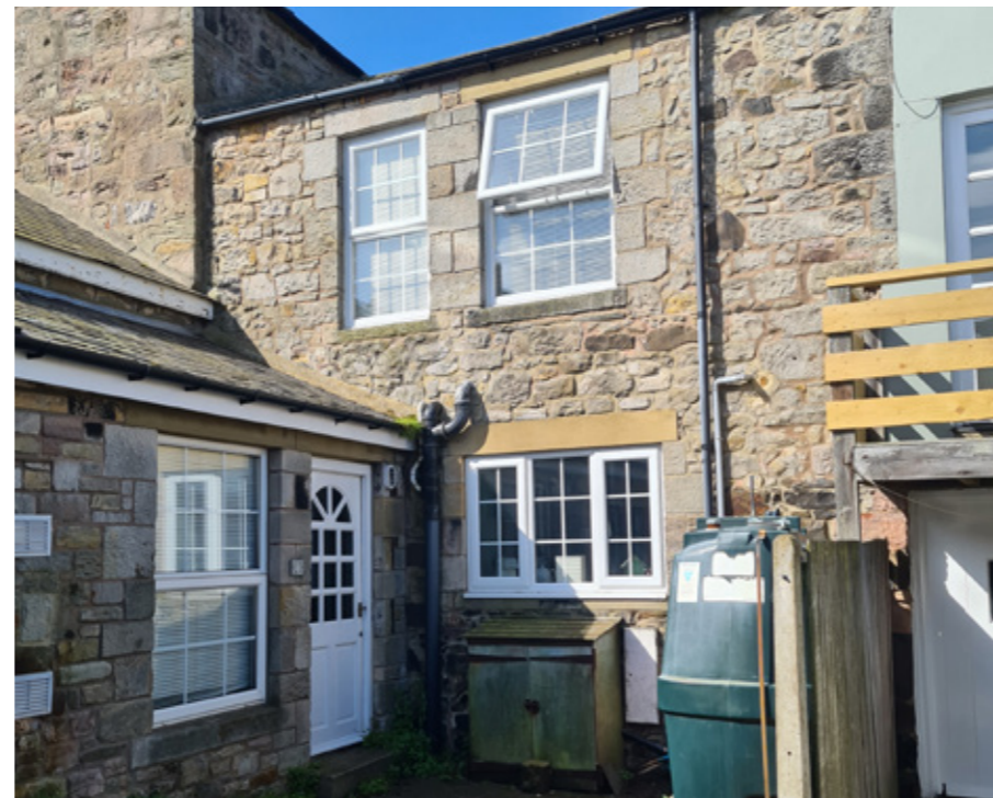
Fig 27. Unoriginal uPVC windows to be replaced with operational timber sash windows with double glazed conservation type units.
