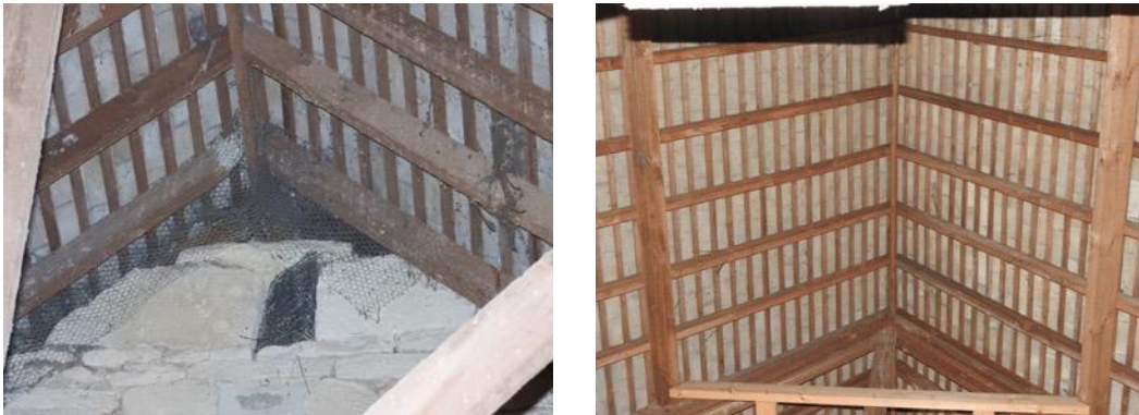
Figs. 13 & 14 Cobwebbed ridge and gable end
