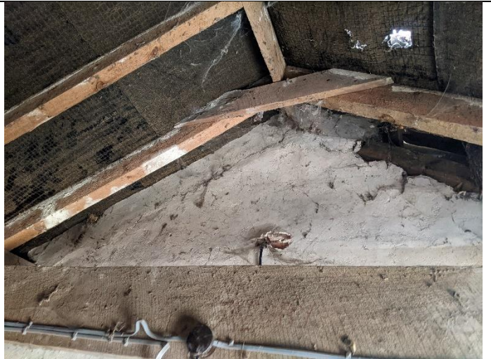
Photo 4 Cobwebby ridge and holes in roof
