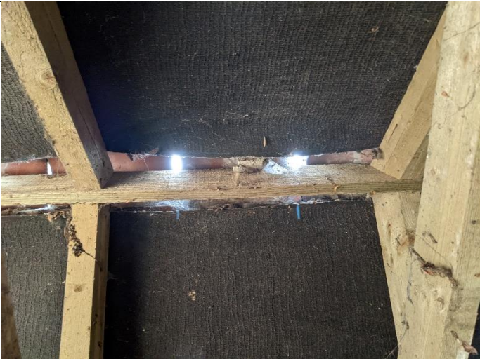
Photo 5 Holes in the ridge
