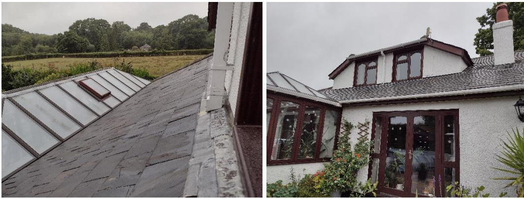
Figure 2: Roof tiles in the proposed works area. Figure 3: Lifted roof tiles around chimney
