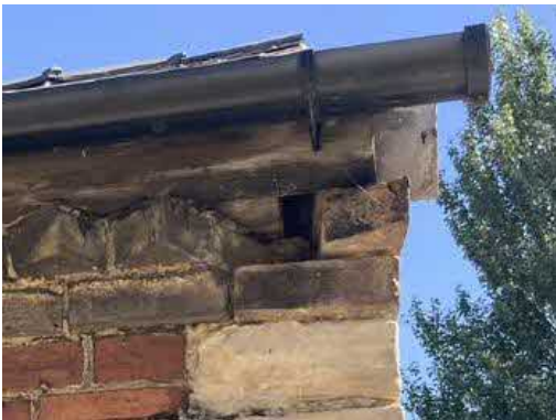
Photograph 7: Gap in brick wall.
