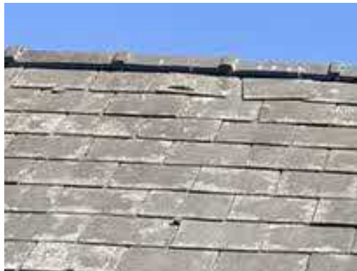
Photograph 8: Small gaps between tiles.
