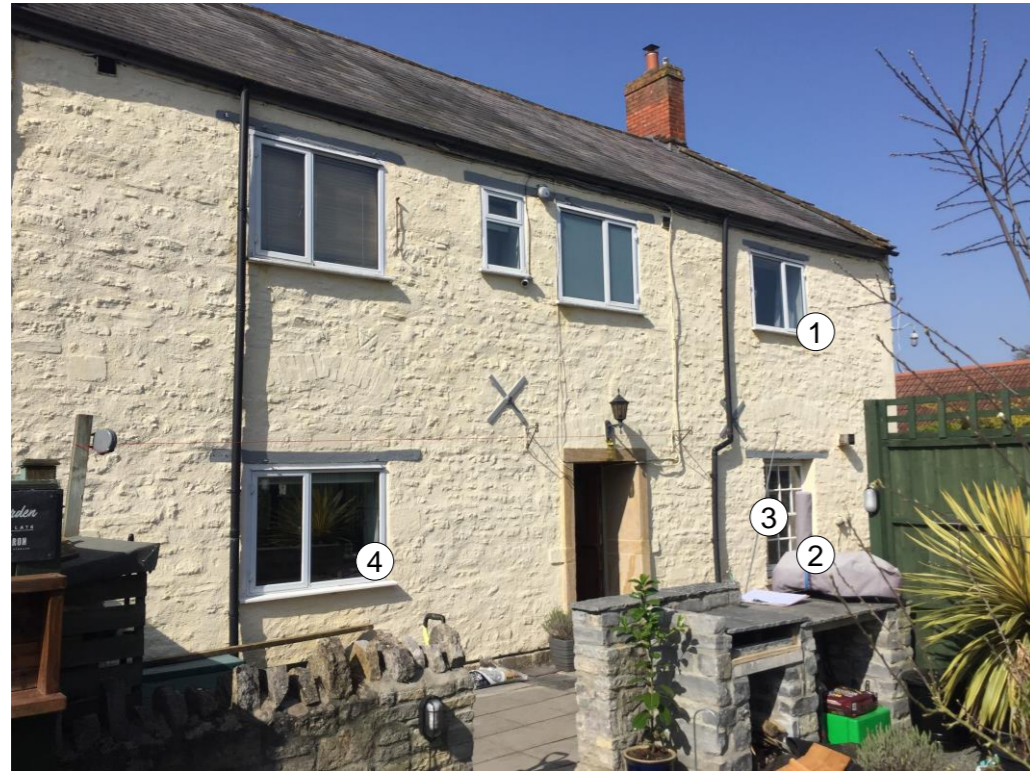
Existing East elevation (rear) of the dwelling showing the 6no. windows to be replaced.
