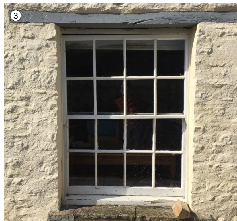
Cill to be raised and window widened to match the existing size of other ground floor window on the East elevation, with existing stone cill to be retained at new height.
