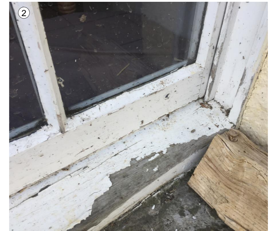
Current deterioration of paintwork and condition to sash window. (Exterior)
