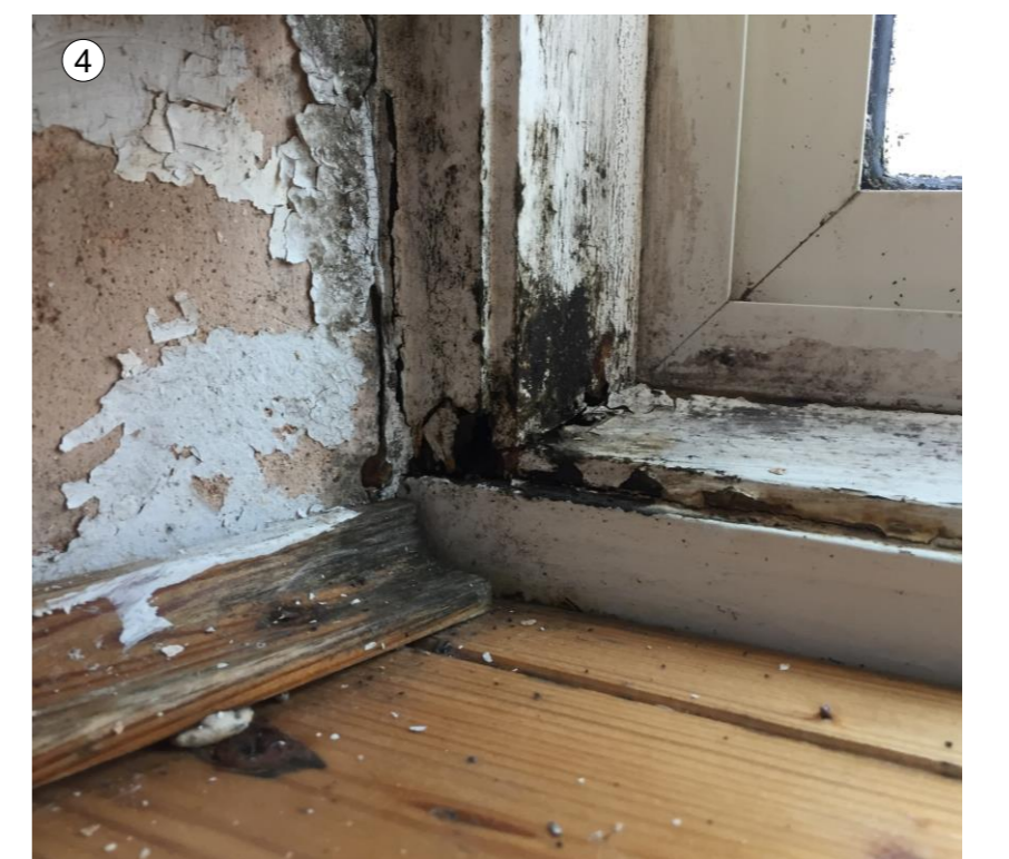
Current deterioration of paintwork showing signs of damp and mould damage to timber frame of uPVC casement window. (Interior)
