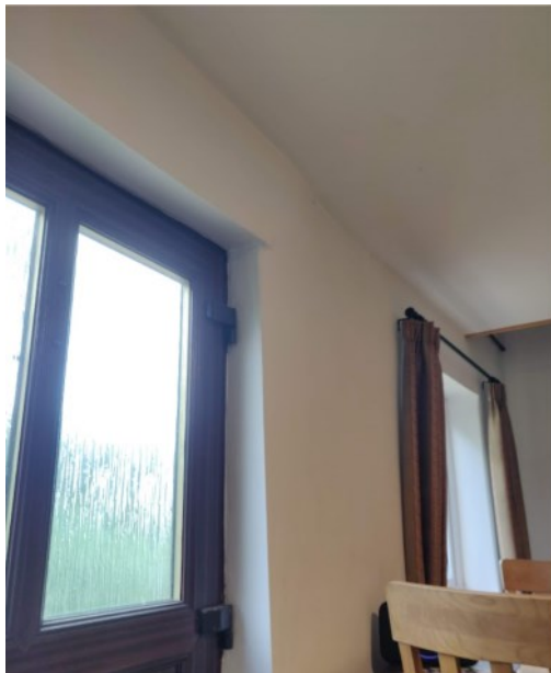
Shows outward leaning wall
