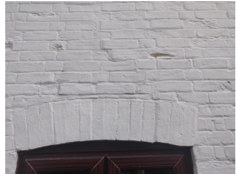
Dropped arch and bulging wall
