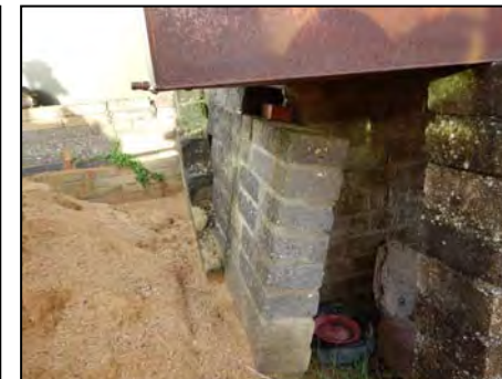
Photo 52 Wall Collapse Beneath Diesel Tanks in North of Site
