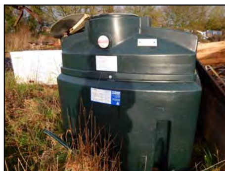
Photo 30 Empty Bunded 2,500L Oil Tank in Centre of Site
