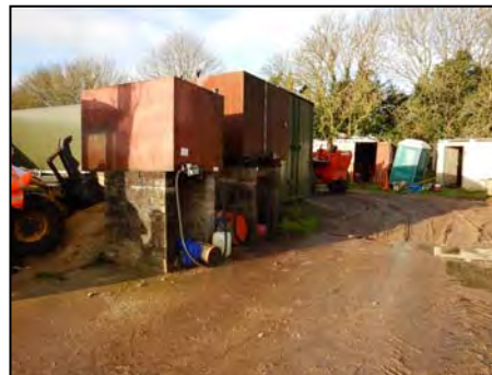
Photo 51 Diesel Tanks in North of Site, View West
