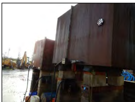
Photo 45 Single Skin Diesel Tanks in North of Site, View South
