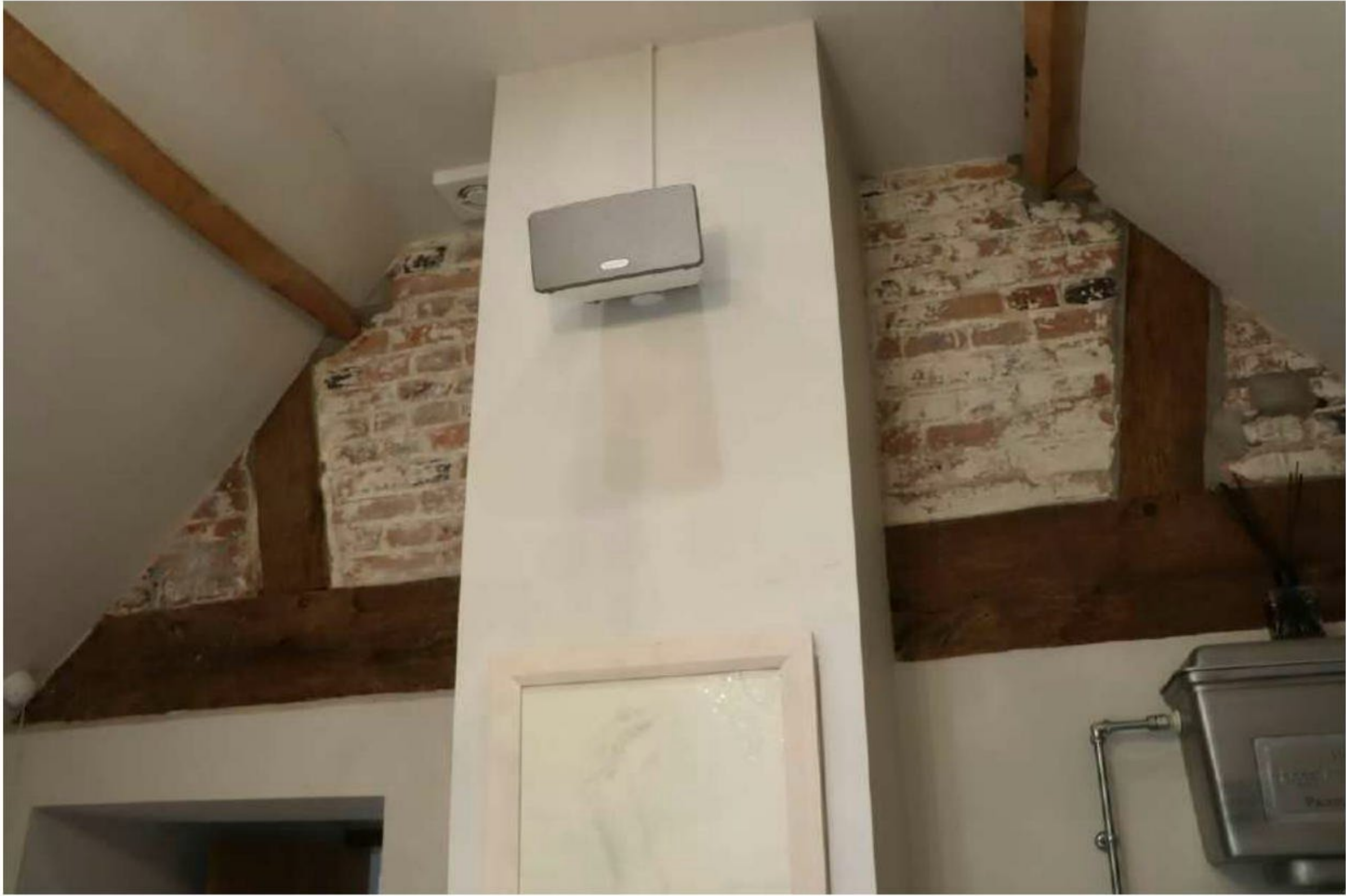
Plate 33: F4: chimneybreast and exposed truss struts in NE gable end of main range
