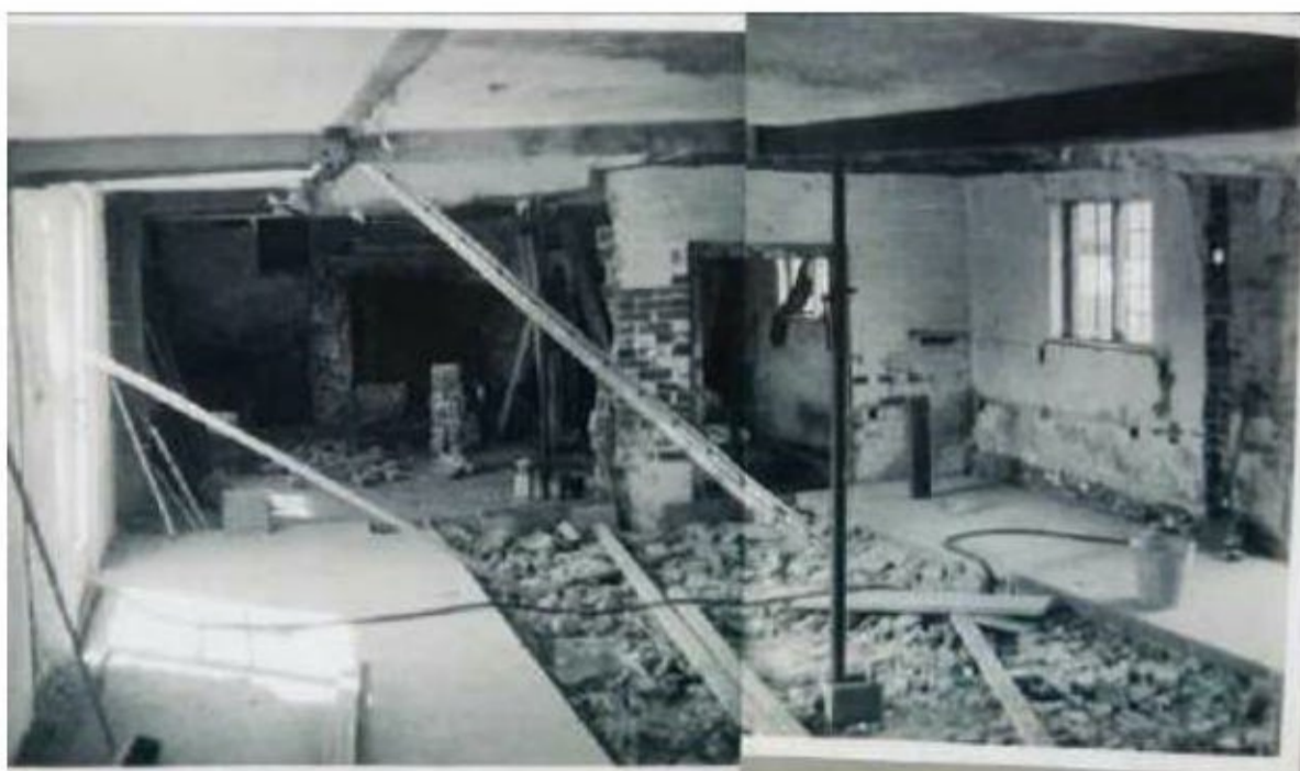
K1: Looking SW from G4 across central bay into G3. A partly demolished brick wall divides central bay from G3. The old staircase (removed) ascended from L to R where the rest of the brick wall has been demolished
