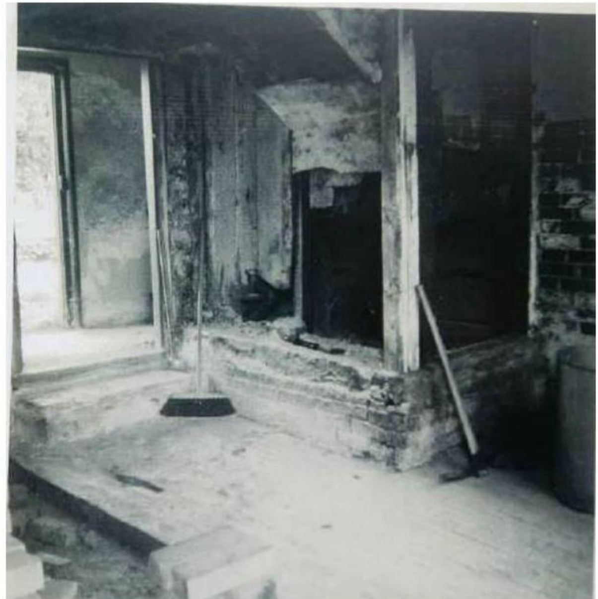
B1: Looking SE across central bay towards partly demolished staircase enclosure (rear entrance to left)
