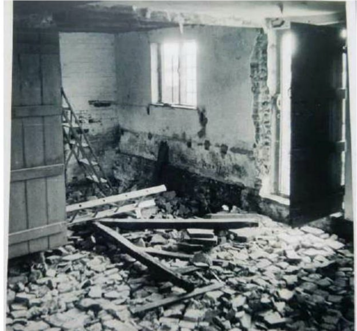
F1: Looking SW from G4 to back door through where demolished wall between G4 & the central bay stood, & into the central bay: the brick floor has been dug out (the person in Photo D1 above is sitting just L of the door in this image)
