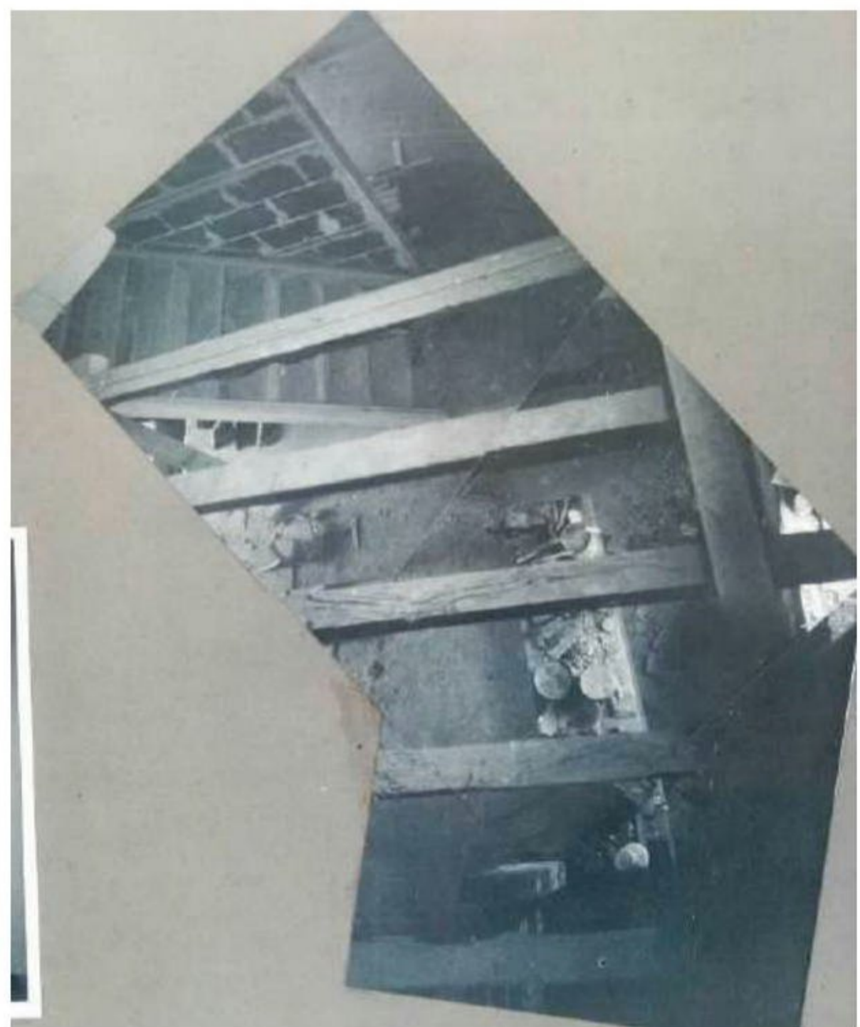
H2: Looking down from F2 into central bay: new staircase, or a temporary one, can be seen against new blockwork wall
