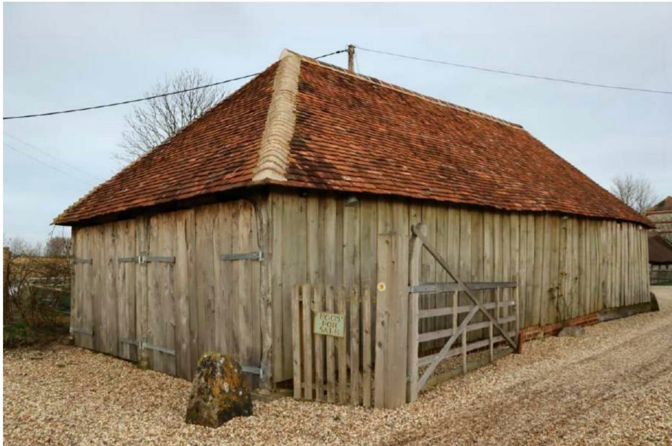
Plate 41: The Grade II listed cartshed restored in 2016 (Building A) – W end with cart entrances and long S elevation
