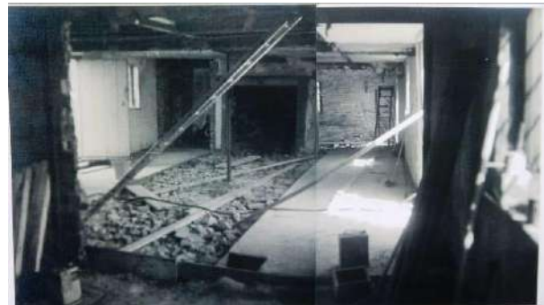
M1: Looking NE from G3 through partially demolished wall where staircase has been removed in central bay across into G4
