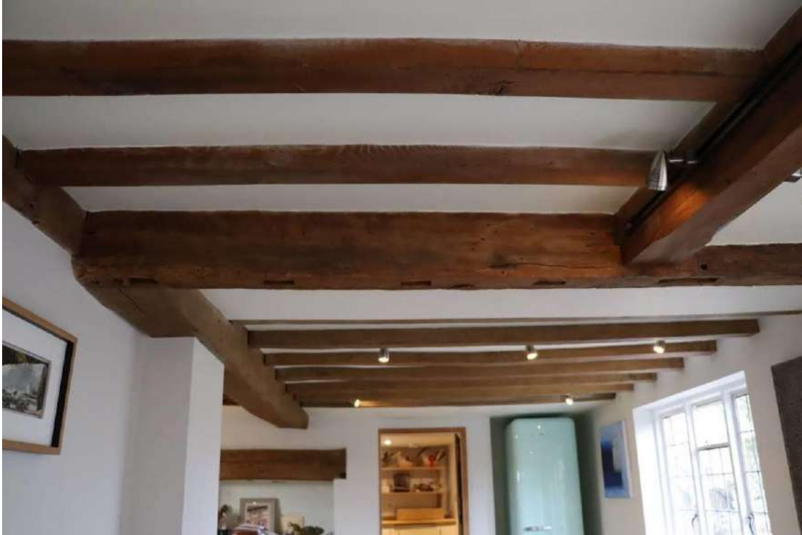
Plate 13: G4, looking NE from central bay into NE bay: the beam with empty mortises across the centre of the image marks the position of the original timber-framed wall dividing the bays; the chamfered and stopped beam joining it to left marks the original extent of the space in the NE bay, while the chamfered beam to right was inserted in the 1950s
