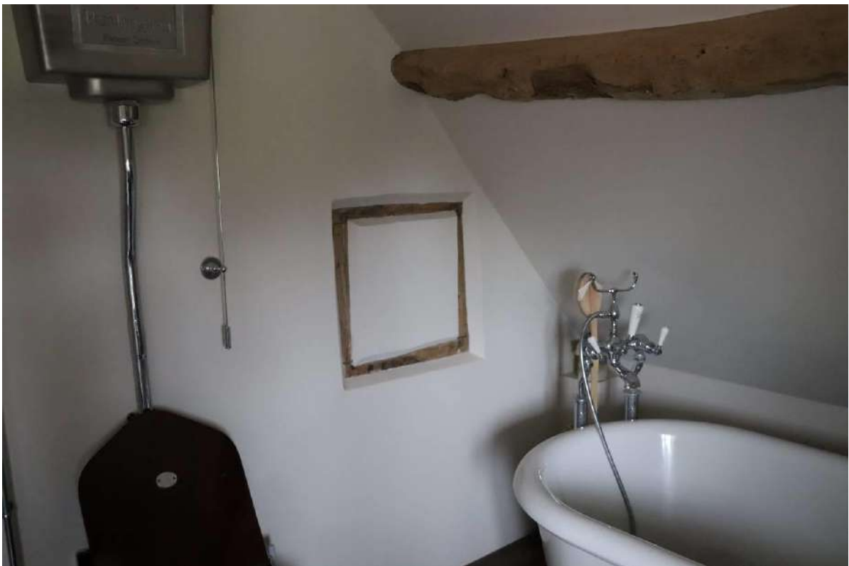
Plate 34: Blocked former window opening in NE gable end of main range, seen in F4
