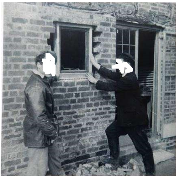
U: Inserting window in new opening in rear elevation adjoining new Crittall French doors
