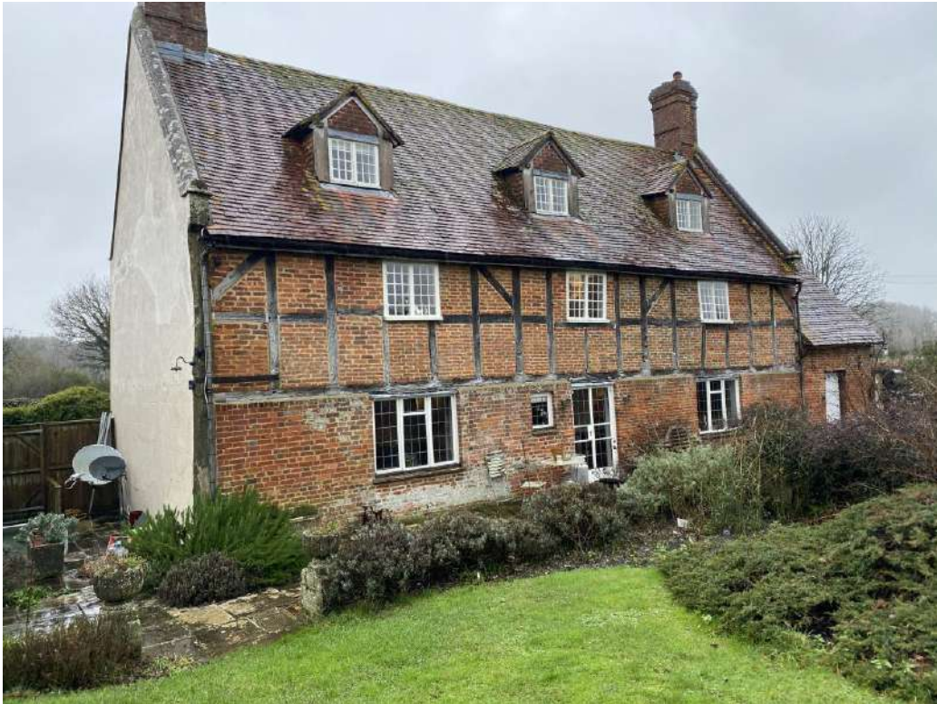
Figure 3: South East facing elevation – proposed link to attach to rendered gable wall
