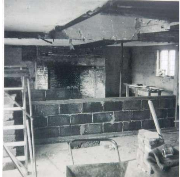
L1: Similar viewpoint to K1 above, looking SW into G3, but from within the central bay: the brick wall is in the process of being replaced with the new concrete block wall
