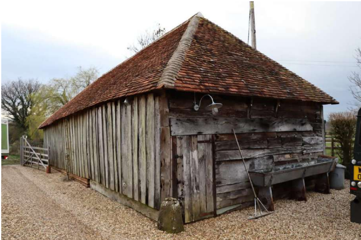
Plate 42: Cartshed (Building A) – long S elevation and E rear end – the building appears originally to have extended further E
