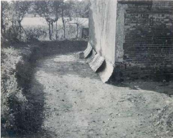
Y: SW gable end, showing where earth bank was excavated away from the side of the building
