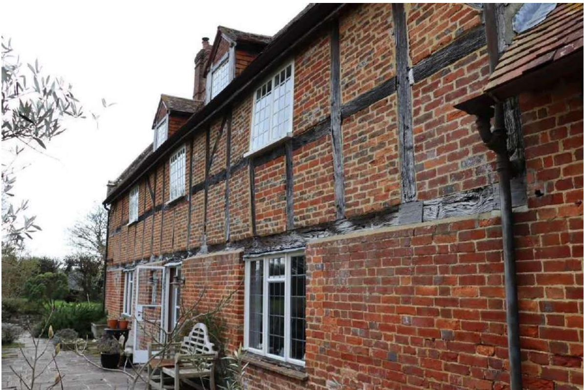
Plate 8: Rear elevation; note projection of ground-floor brickwork from the original building plane, with enlarged window opening in foreground and French doors
