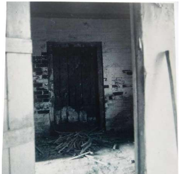
V1: Old double-thickness door in undetermined location. The nature of the brickwork suggests somewhere in the central bay.
