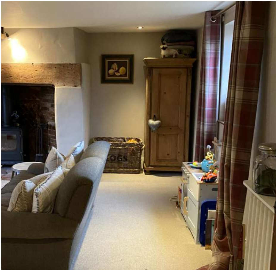
Figure 4: Internal view of existing gable wall where existing window opening (currently blocked in) is to be altered to form a doorway opening to link.
