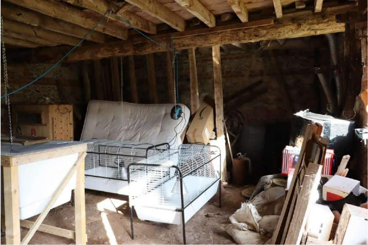
Plate 51: Building C – interior, looking E towards former partition in E end bay, and ladder to hay loft
