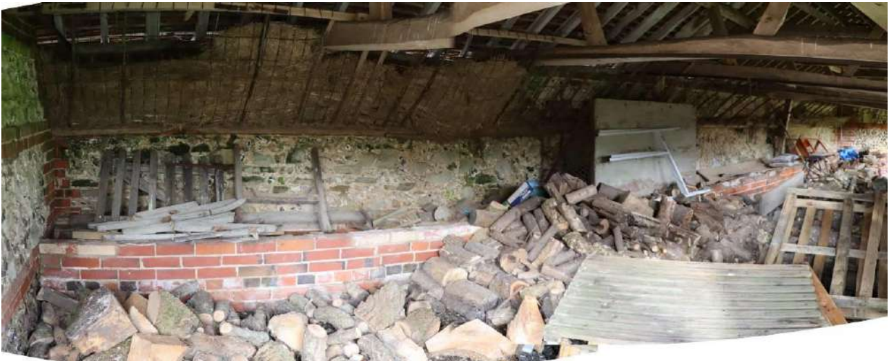
Plate 48: Building B – interior, looking to rear wall with feeding trough and manger
