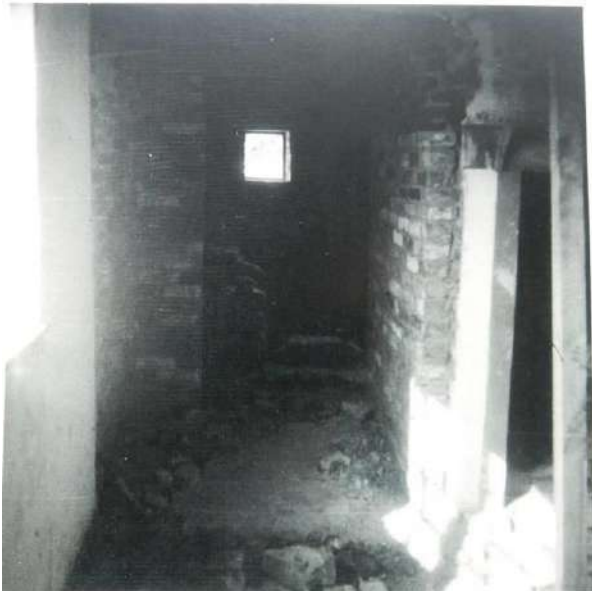
T1: Following demolition of bread oven, looking NE from G4 into G5 in 'brewhouse' addition
