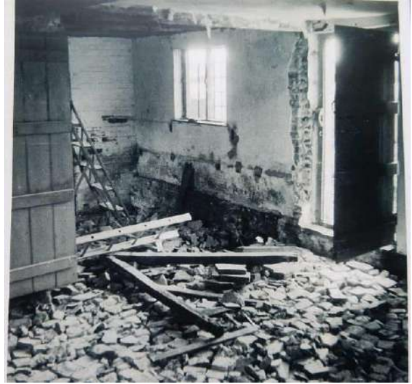
F1: Looking SW from G4 to back door through where demolished wall between G4 & the central bay stood, & into the central bay: the brick floor has been dug out (the person in Photo D1 above is sitting just L of the door in this image)
