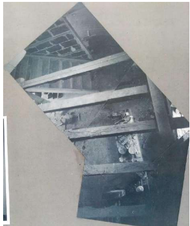
H2: Looking down from F2 into central bay: new staircase, or a temporary one, can be seen against new blockwork wall
