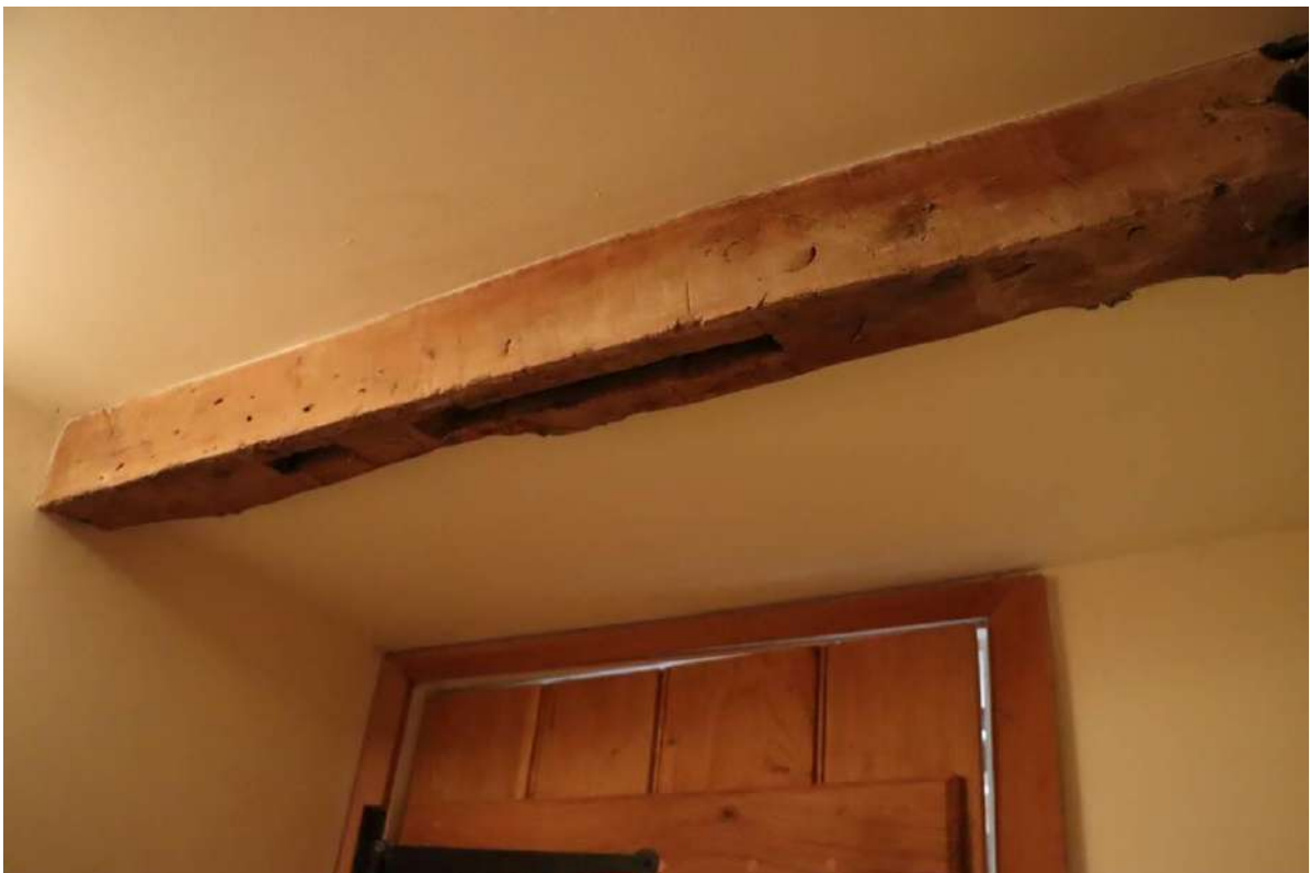
Plate 12: G1: original beam with empty mortises from the removal of the timber-framed wall dividing the northern from the central bay
