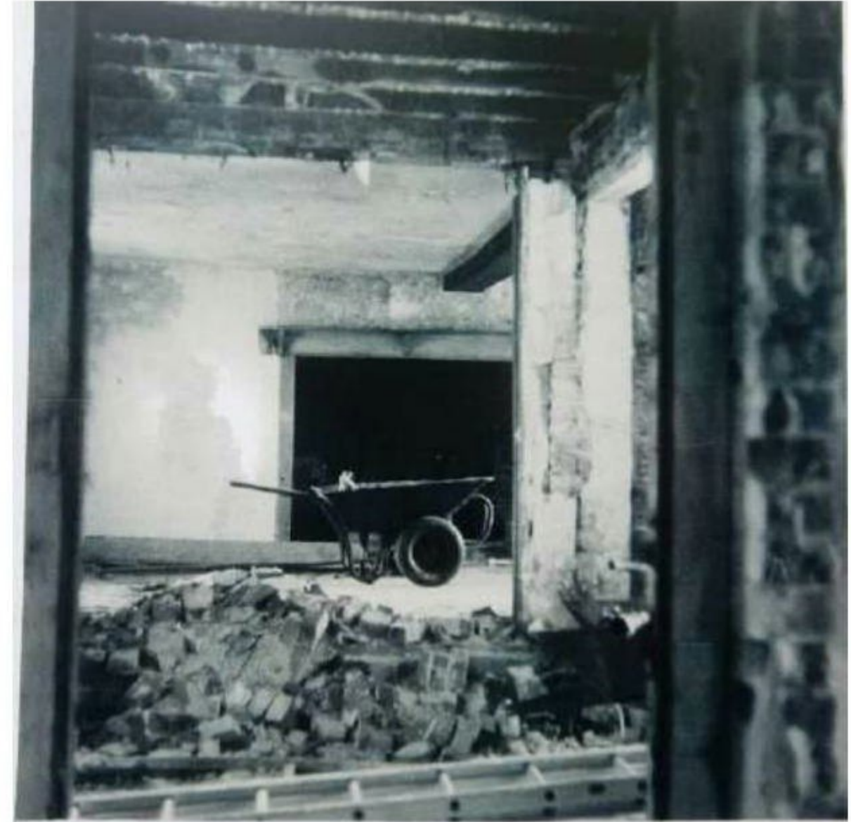
Q1: Looking NE from G3 across central bay into G4; note wall left of G4's fireplace, behind which was a bread oven
