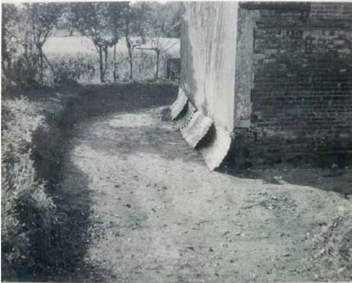
Y: SW gable end, showing where earth bank was excavated away from the side of the building
