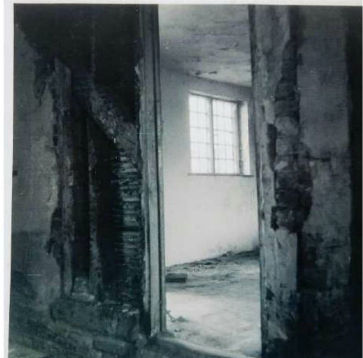
G1: Looking N from central bay into G4 (the timber-framed wall was yet to be demolished)
