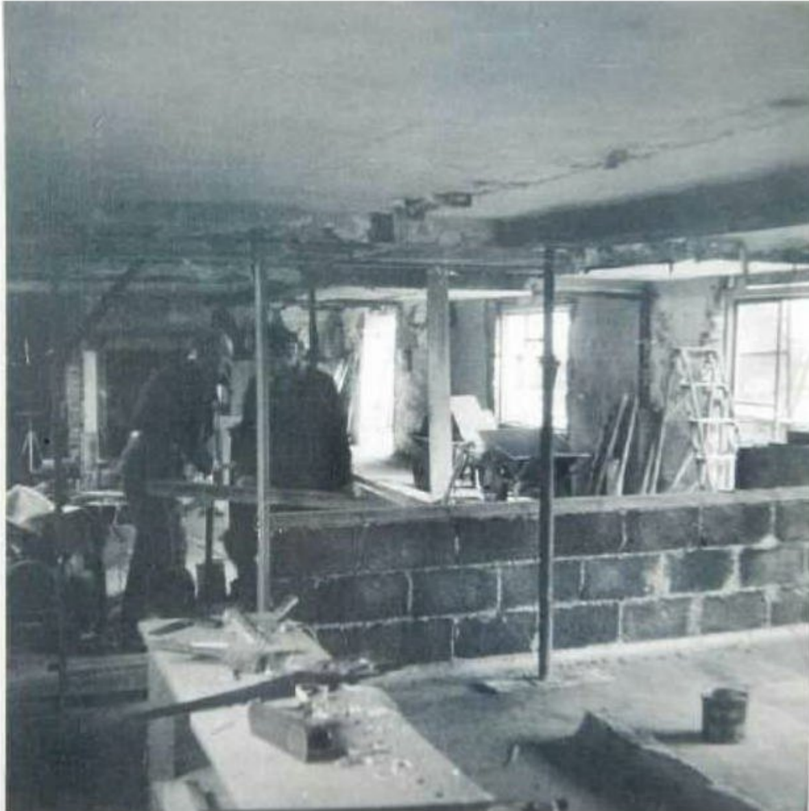
O1: Looking NE from G3 across central bay into G4: new concrete blockwork wall being built to divide G3 from central bay
