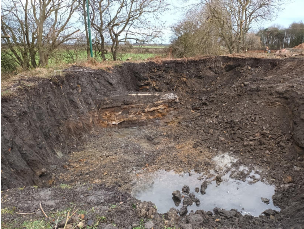
Plate 1: View east showing edge of curtain wall. Note depth of colliery spoil and crest of slope to left of picture.
