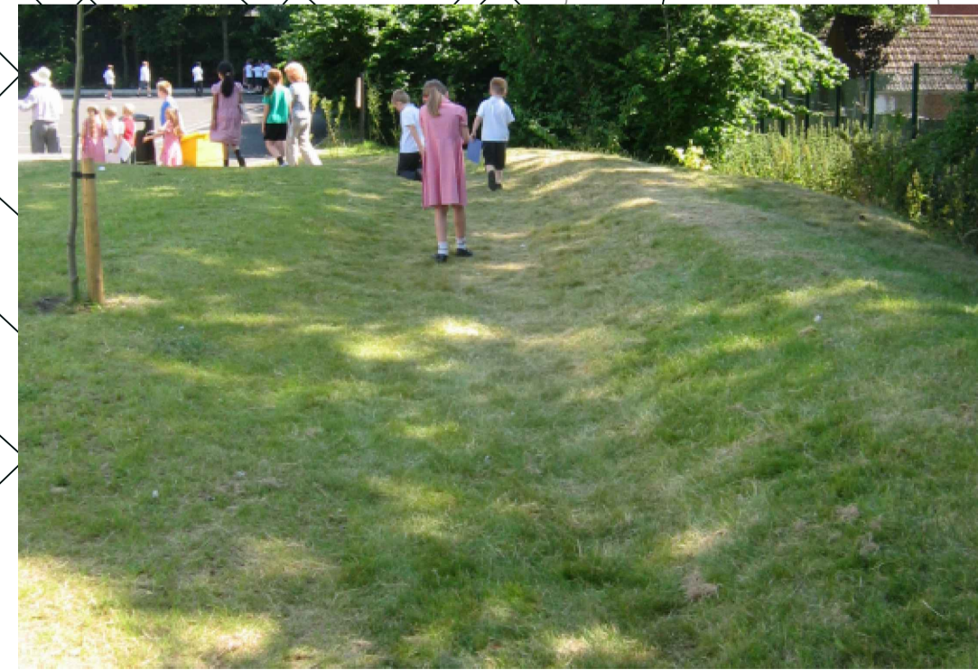
SHALLOW GRASSED SWALE EXAMPLE IMAGE REFER TO MAYOR OF LONDON REIMAGINING RAINWATER IN SCHOOLS REPORT
