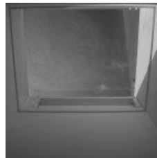
An internal view of the natural ventilation louvre turret from inside a classroom
