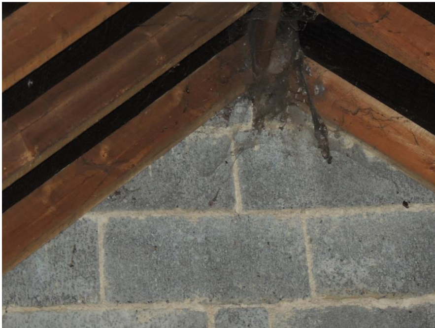
Photo 13: Note cobwebs at apex of gable wall
