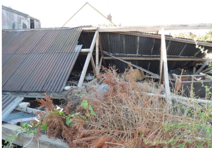
Photo 17: Part of the building had collapsed since the earlier survey
