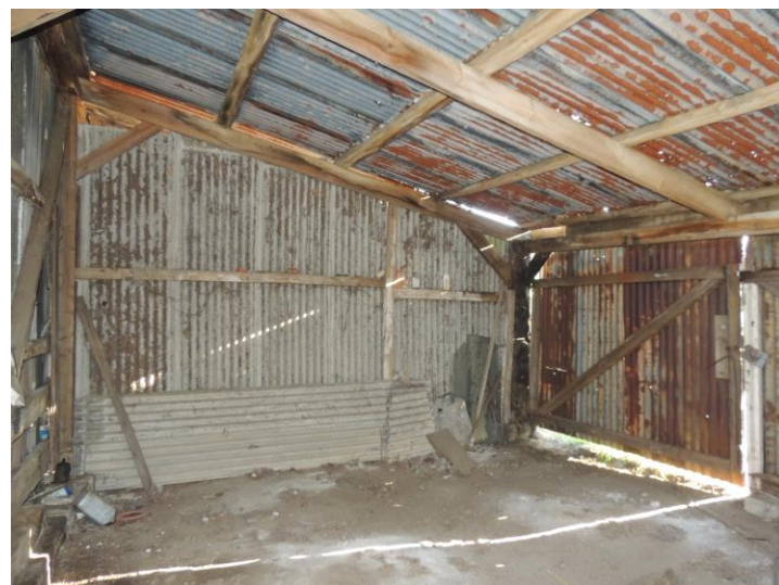
Photo 15: The interior of the shed had no features that might be occupied by bats
