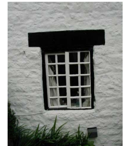
2022 Example of Horizontal sliding sash window to the Annexe (Photograph: Author's own)
