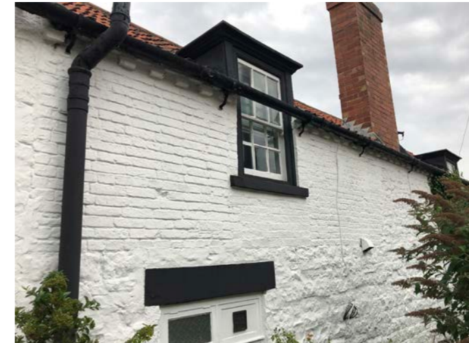
2022 Front of The Cottage showing varying infill areas of brickwork. (Photograph: Author's own)
