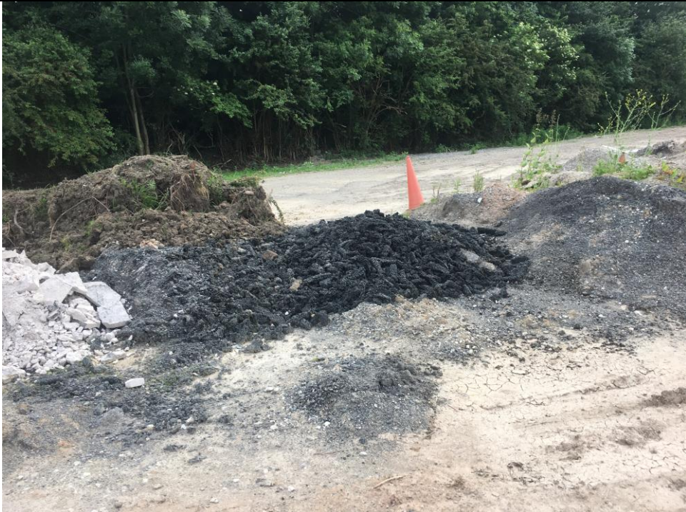
No 9 | Broken tarmac within the stockpile (No 8).
