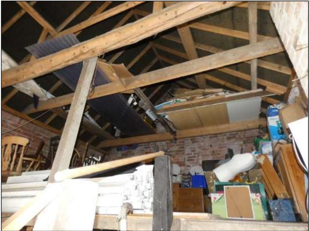
Photograph 1.5 : Internal view of the mezzanine hayloft in the western half of the building, above the area shown in photograph 1.4 above, and the roof structure.
