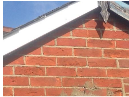
Photograph 6: Eastern elevation. Extension to be added here. Soffits are in good condition with no gaps.
