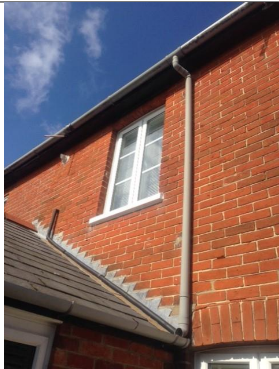
Photograph 3: well-sealed roof tiles, soffits and lead flashing on current first floor extension – new extensions to be added here on ground and in part on second-storey level.
