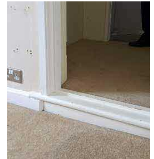
Uneven first floor levels.
