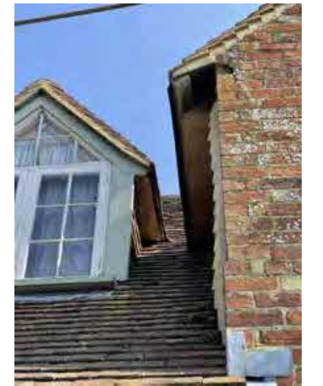
West: poor detailing
