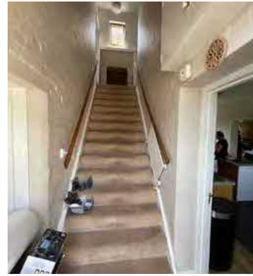
Narrow, steep & tall inaccessible staircase.
