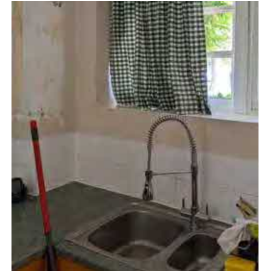
Kitchen: inadequate storage & tired.
