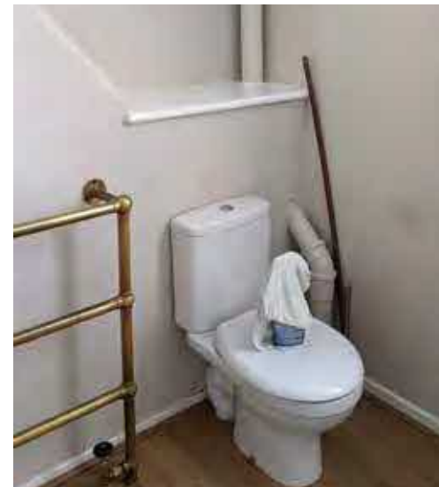
Impractical facilities, exposed pipes.
