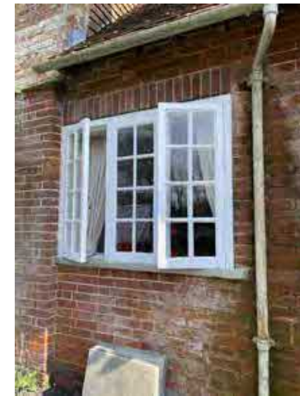
West: leaking downpipes
