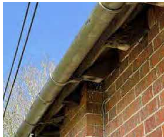
Shifted rafter ends & loosened brickwork
