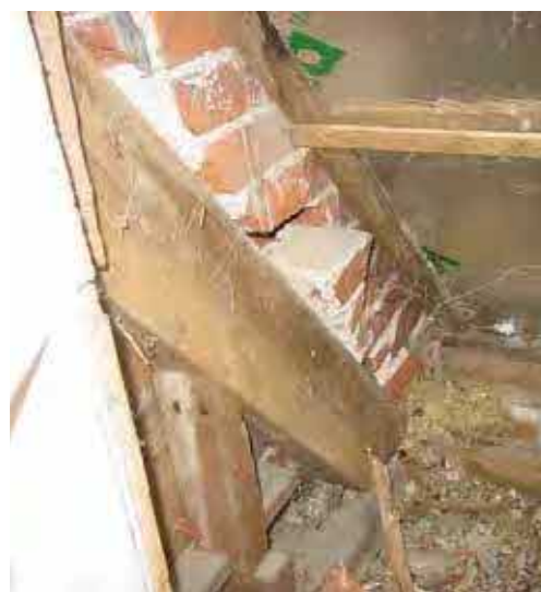
Displacement & daylight in roof space.
