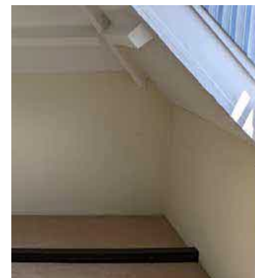
Unsupported cut purlins, ties above floor.
