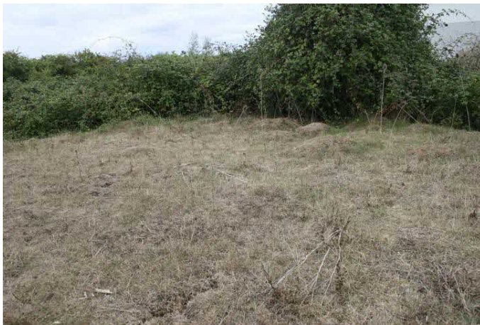
Photo 2: Dried vegetation on thin soil above concrete cover of reservoir plus anthills
