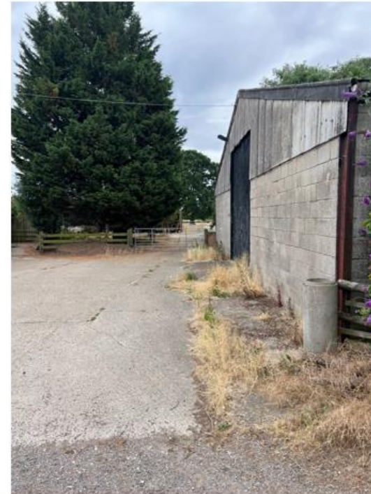
Photo No.2: Facing south showing the eastern face of the building proposed to be converted
