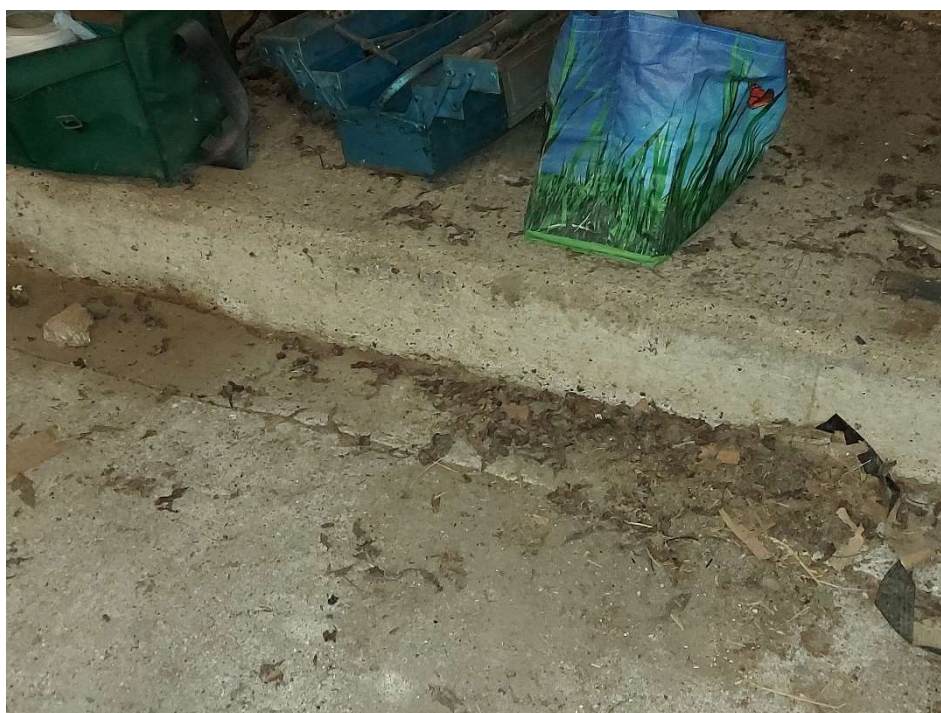
7.12 General view of existing internal slab and plinth upstand to South elevation of barn
