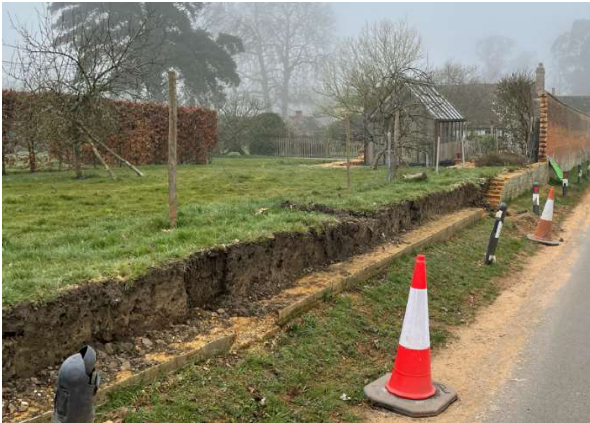
Fig 4. Collapsed wall close-up along Bottle Lane
