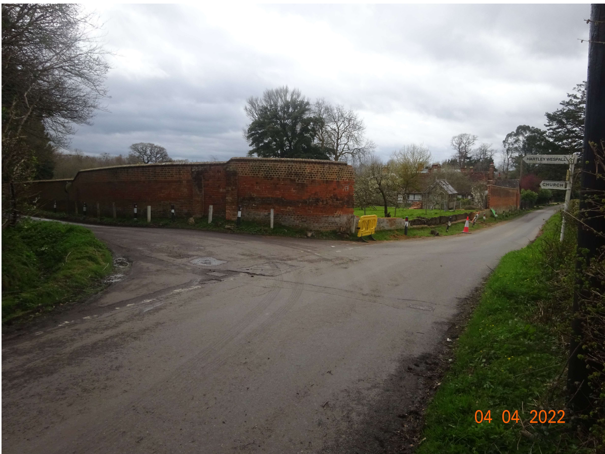
Fig 2. Overall elevation of collapsed wall between Turgis Green Lane & Bottle Lane
