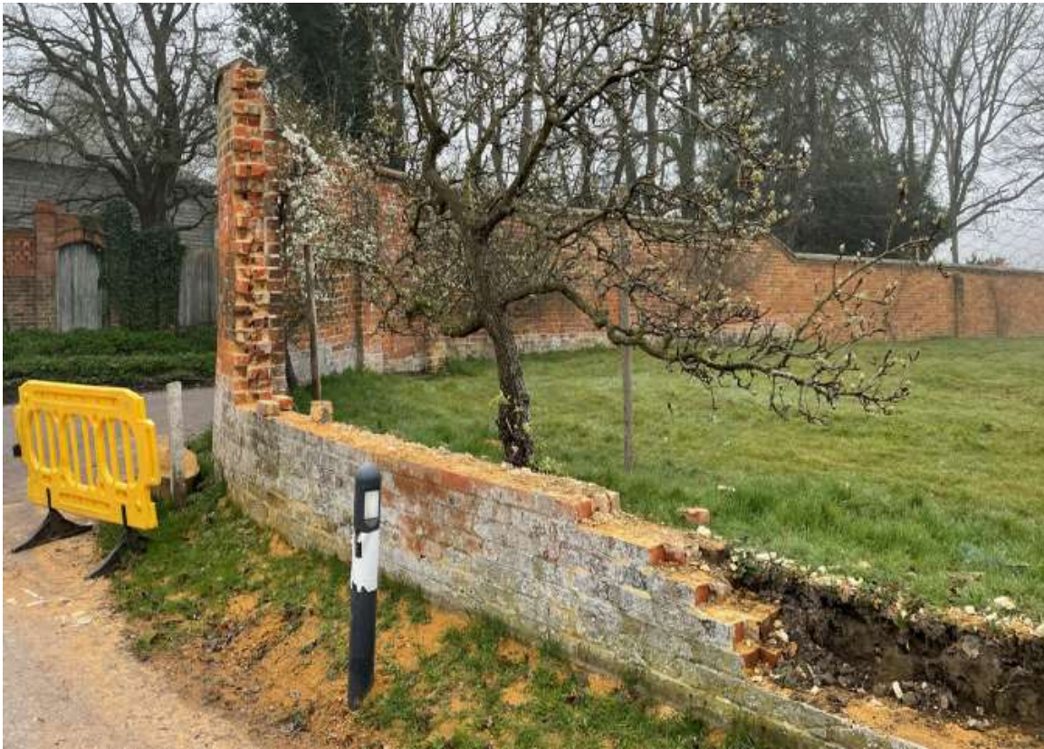
Fig 3. Collapsed wall close-up nearer Turgis Green Lane corner
