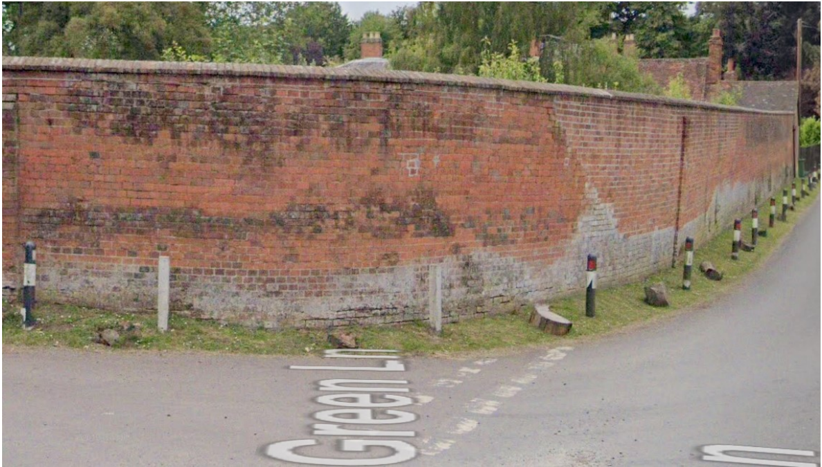
Fig 1. External elevation to original perimeter wall before collapse to Hartley House
