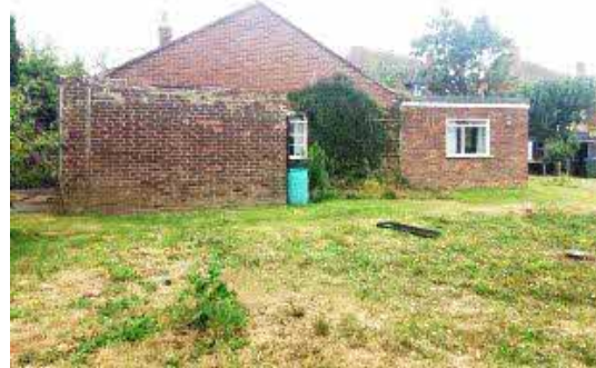
Photo 2. View south of north elevation. Brick and tile construction with metal window frames on this and the rear parts of the house. Note dry lawn around house.
