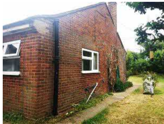
Photo 4. South elevation with uPVC windows. No visible cracks or holes to be exploited by birds or bats.
