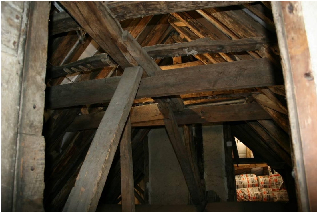
The remnants of the crown post roof looking S over the hall.
