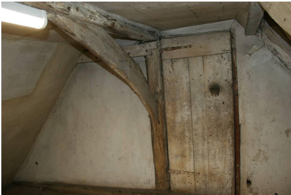
Detail of the crown post and the door into the main roof.
