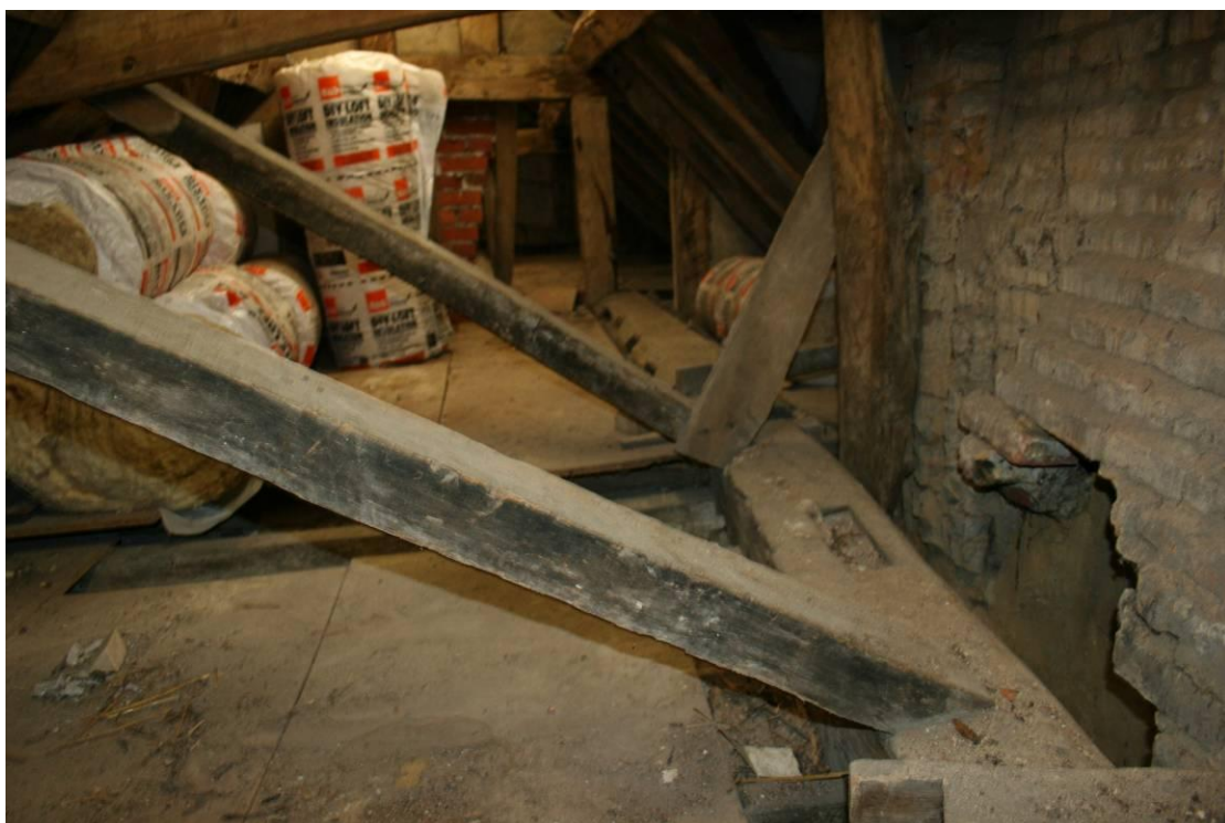
Two reused main beams have been used to make up the ceiling frame.
