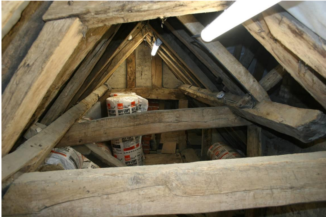
Looking SW in Cross-wing over Bedroom 3. Note the fall of the frame.
