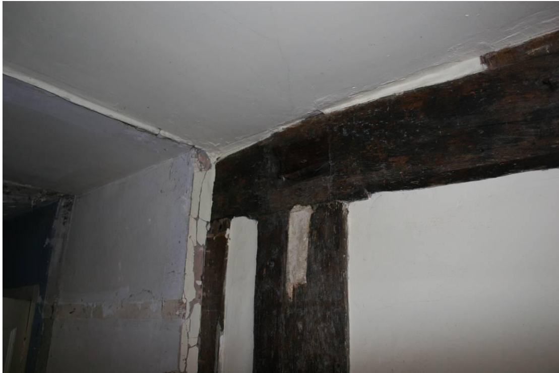
Redundant mortices in the tie-beam and storey post.
