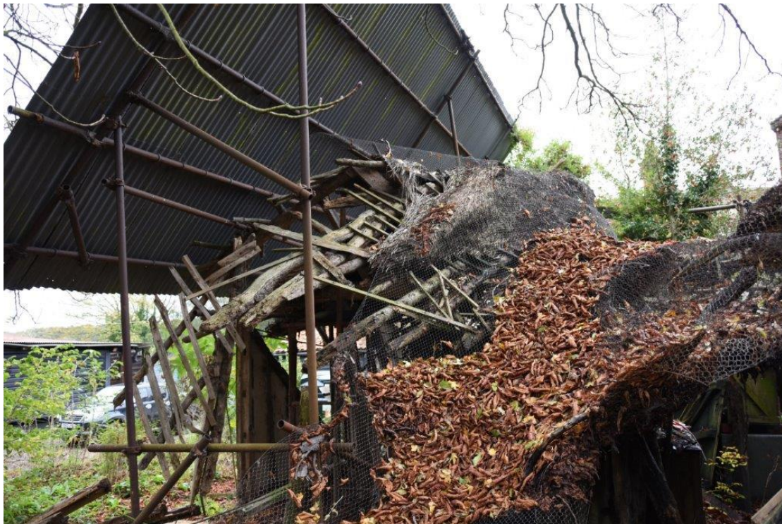
2020. The east elevation of the Summer House before the failed scaffolding was removed.
