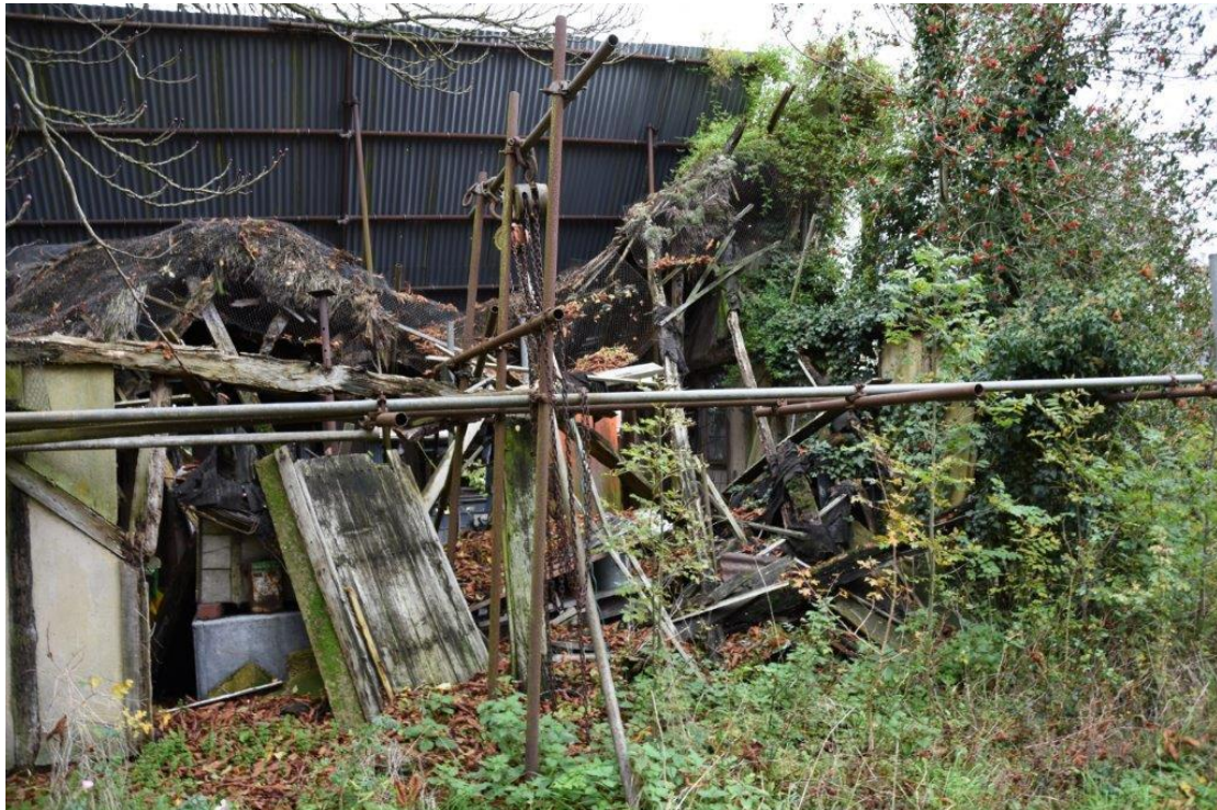
2020. The north elevation of the Summer House before the failed scaffolding was removed.
