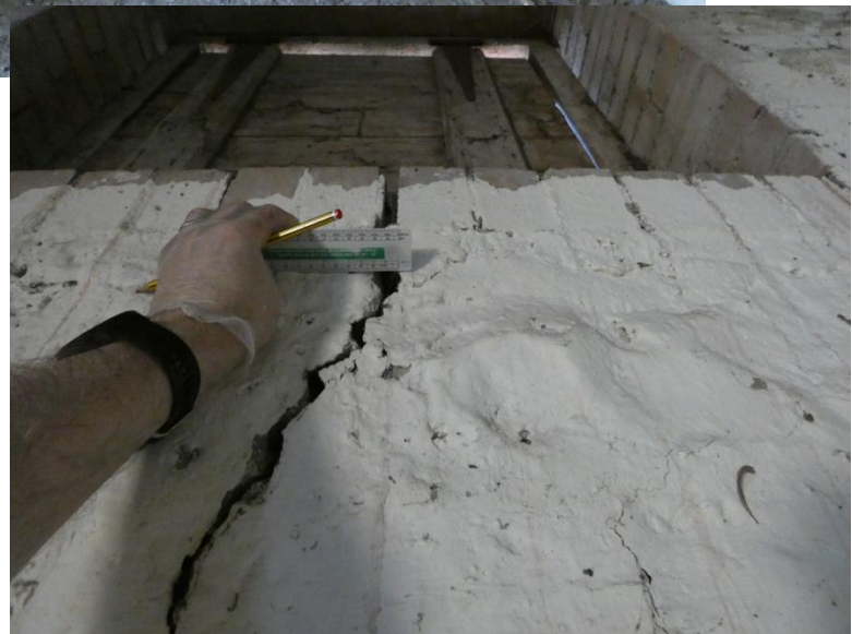
Photo 20 – Barn L interior – North gable of Barn L – Suspected foundation related movement
