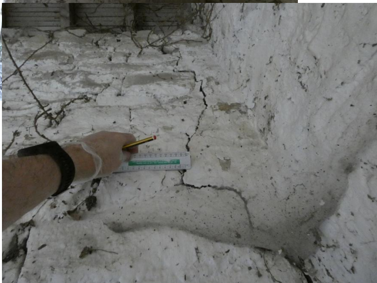
Photo 23 – Looking to north west corner of Barn L – Suspected foundation related movement
