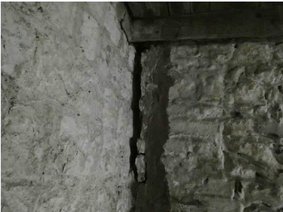
Photo 9, example of a crack in the stonework of the outbuilding on the lower level.
