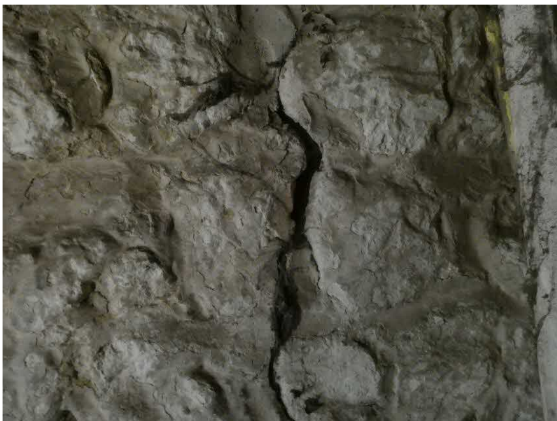
Photo 14, crack in the stonework of the carport.
