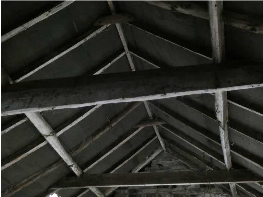
Photo 10, internal view of the upper level of the outbuilding, with bitumen lined roof.
