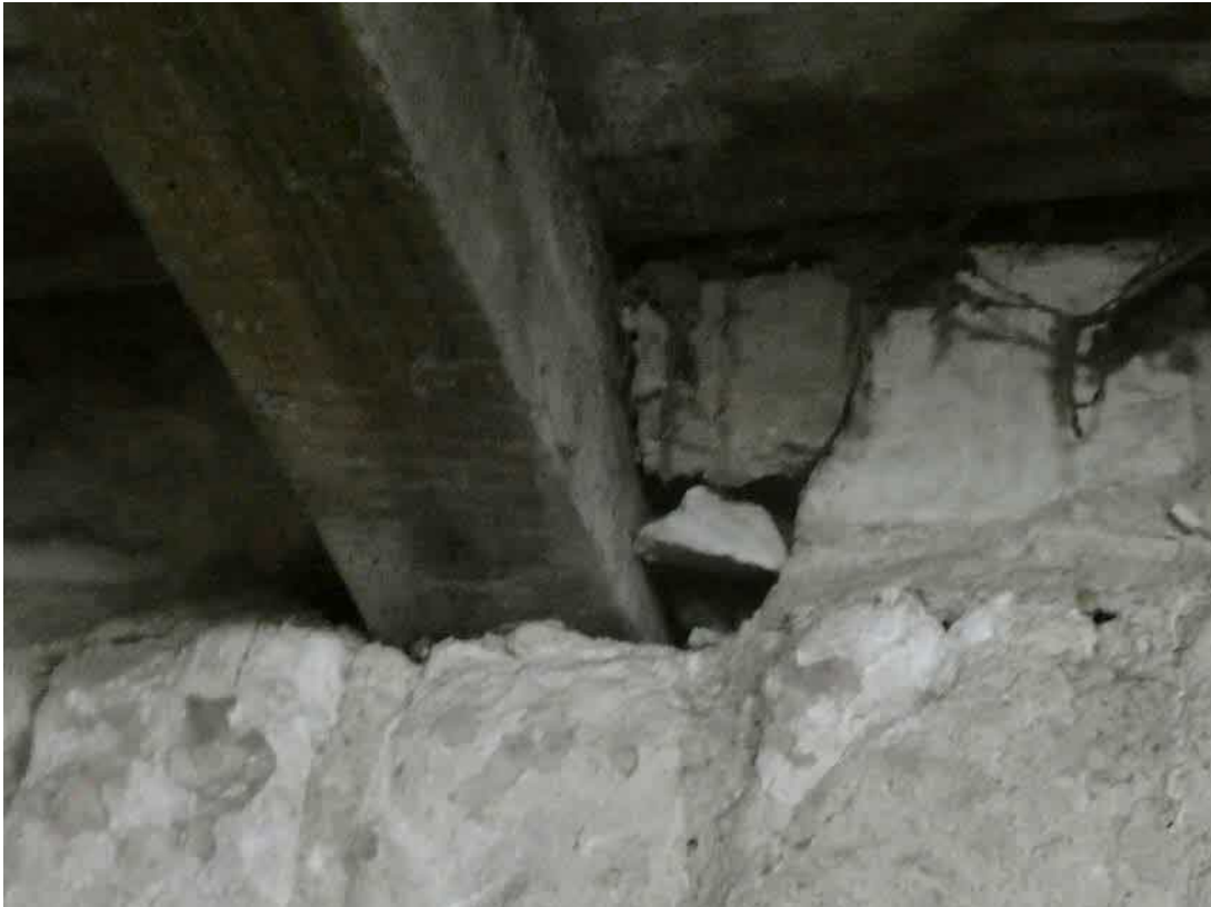
Photo 8, example of one of the gaps around the timber floor joists in the outbuilding which could be used by crevice dwelling bats.
