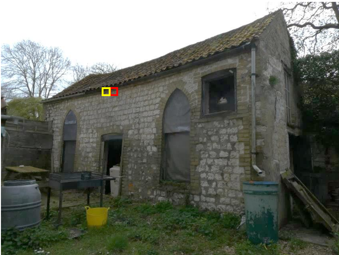
Photo 3 , common pipistrelle and brown long-eared roost location on the north aspect of building one highlighted in yellow and red respectively. 7 th September 2022.
