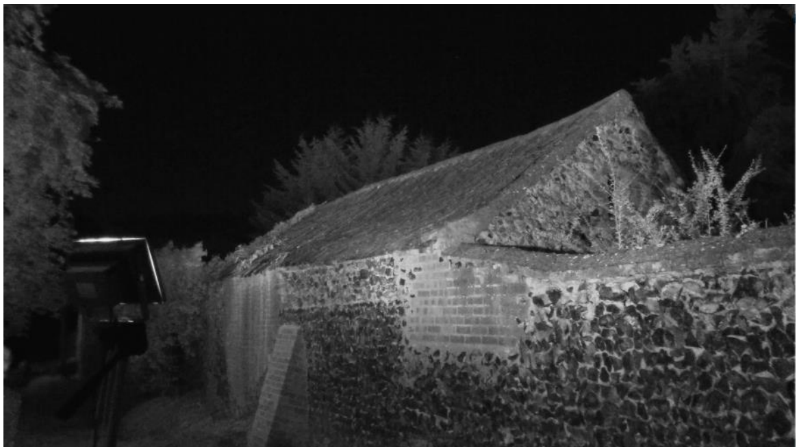
Photo 2 , infrared camera situated on the southeast corner, taken from the darkest part of the survey.
