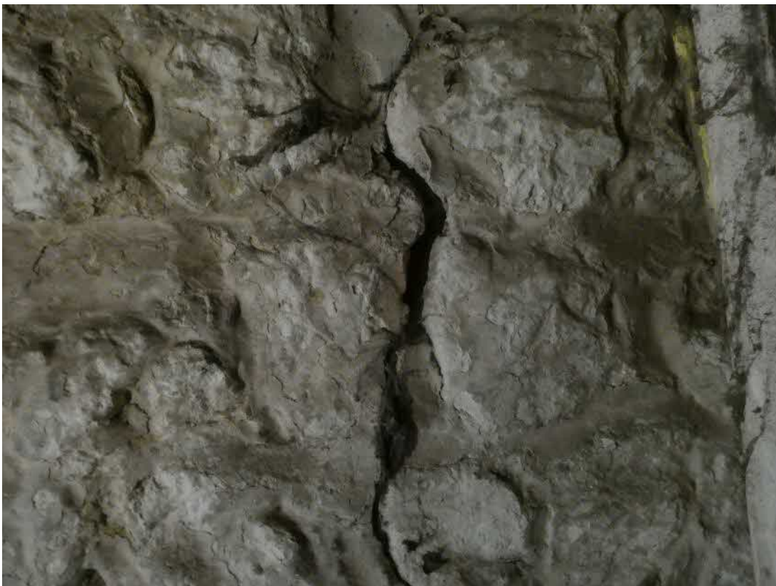
Photo 14, crack in the stonework of the carport.
