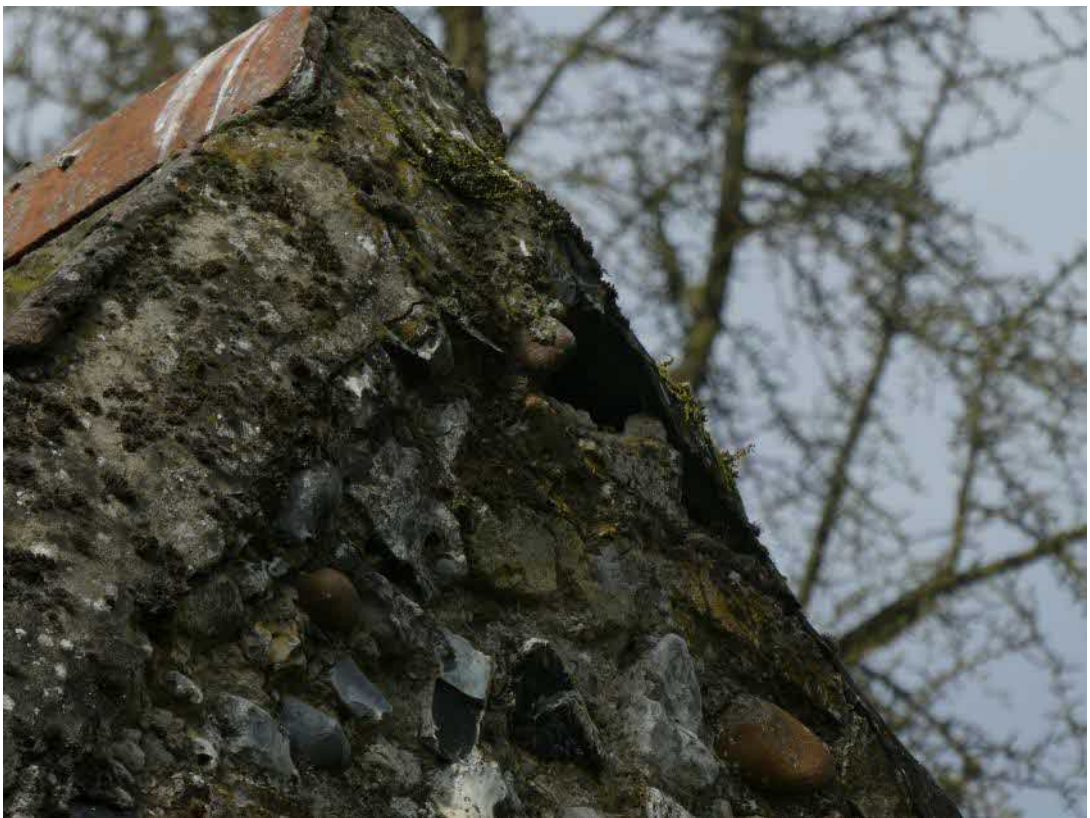
Photo 11, gap at the eastern apex which could be used for access and/or roosting opportunity.
