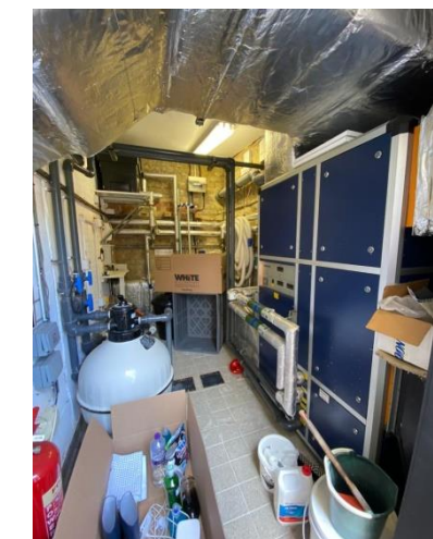
Photo P2.8 Heatstar Phoenix 3000 unit controls the Pool Hall environment and heats the pool
