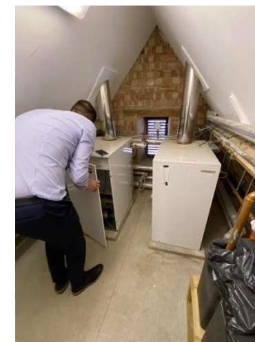
Photo P2.7 Two boilers located in roof void serving the Swimming Pool building
