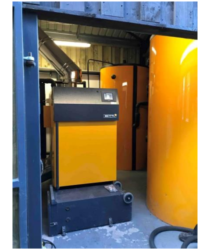
Photo P4.2 Modern biomass boiler plant
