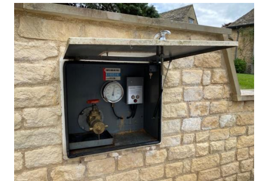
Photo P2.4 Oil fill point in Garage Yard
