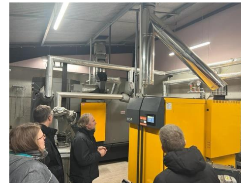
Photo P4.3 A Larger biomass boiler plant
