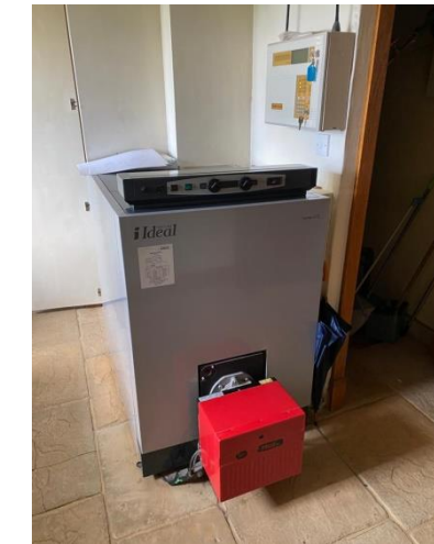
Photo P2.6 Ideal Harrier GTS boiler serving the House
