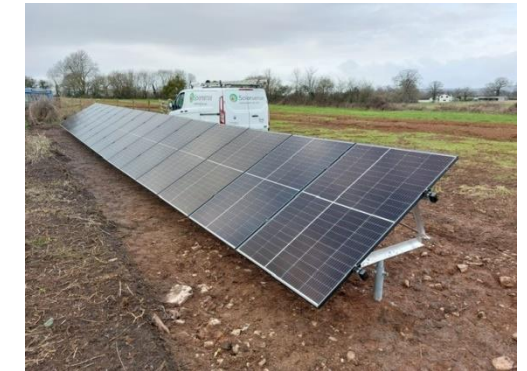
Photo P3.2 Solarsense photovoltaic array
