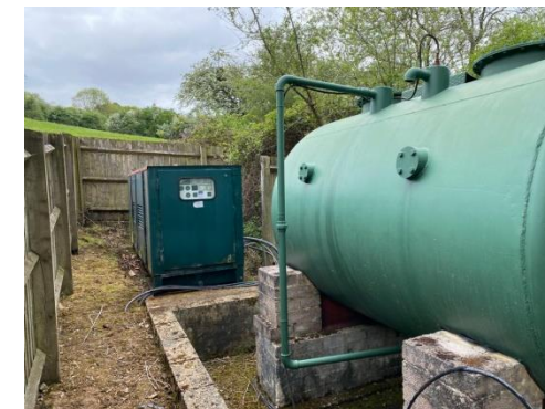
Photo P2.3 Standby diesel generator and oil tank located remotely from the House
