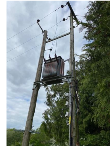
Photo P2.1 Pole-mounted transformer adjacent to Garage Block
