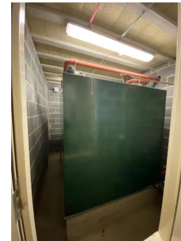
Photo P2.5 Oil storage tank in Garage basement
