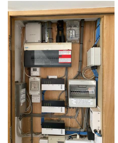
Photo P2.2 Electricity meter and main distribution board in House
