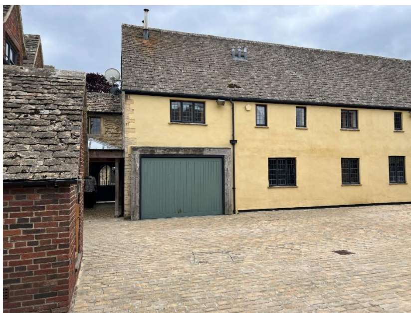
Figure 6. The garage door which is to be modified into a window to match the adjacent windows.
