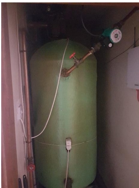
Figure 13. The existing boiler tank in the utility room.
