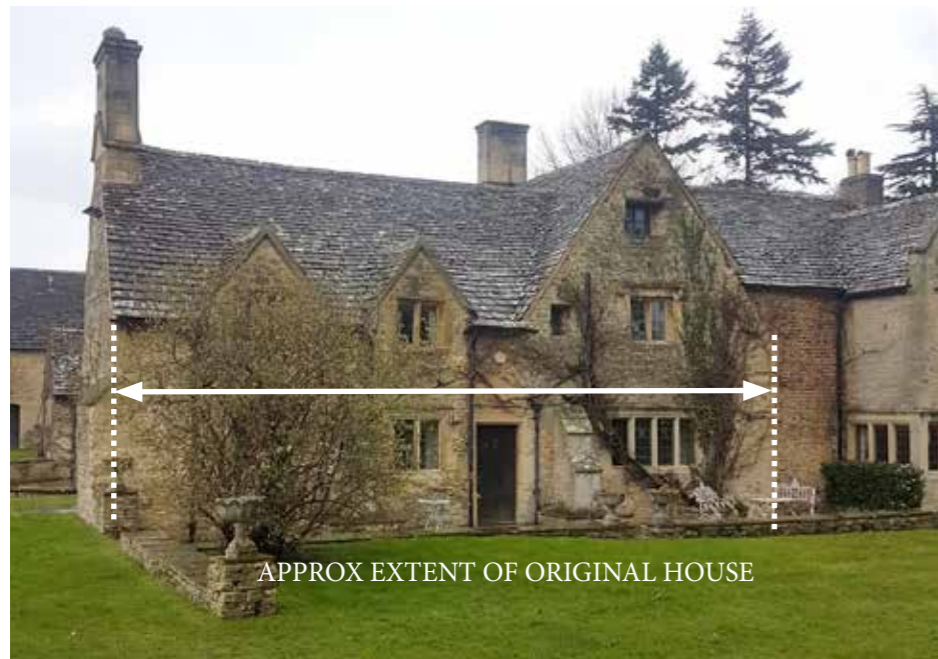
Modern view of part of the southern elevation, with the extent of the original, sixteenth century house indicated.
