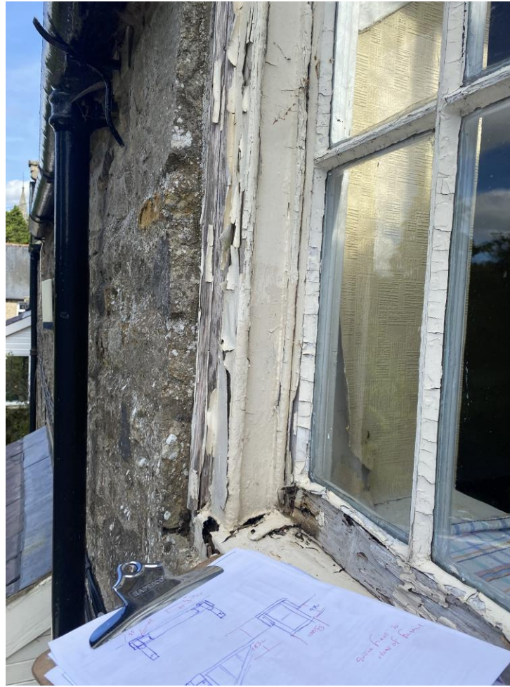
Outer cheek, sill and bottom rail of sash showing decay. Failed tenon joints on bottom sash. Lower section of outer cheek missing.
