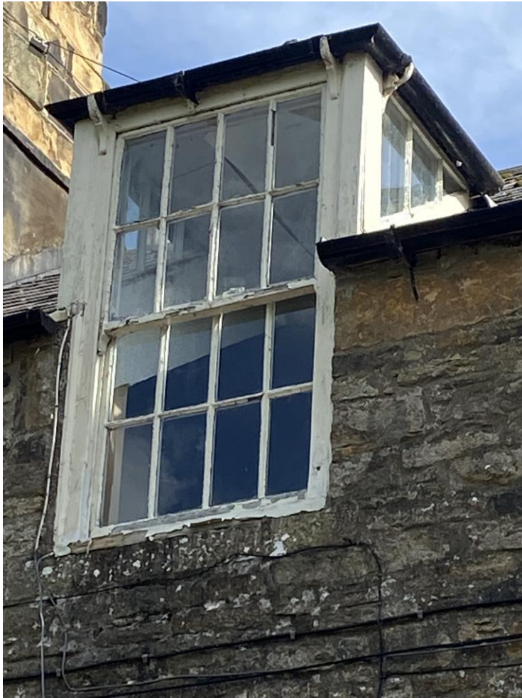
Missing putty on glazing bars has caused water ingress and further damage to glazing bars. Sill has failed due to lack of paint.
