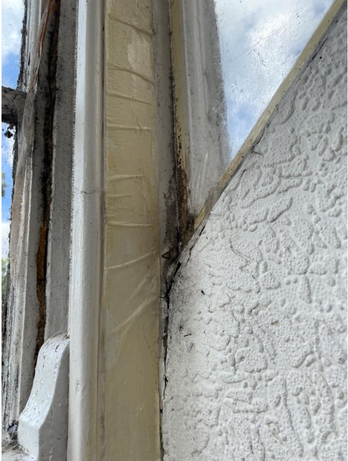
Failed tenon joints to the lower sections of side returns due to water ingress
