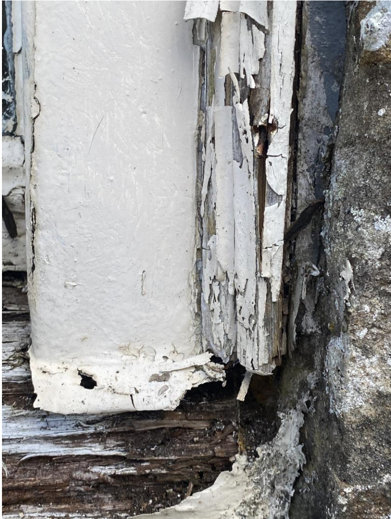
Decayed outer cheek and external sill
