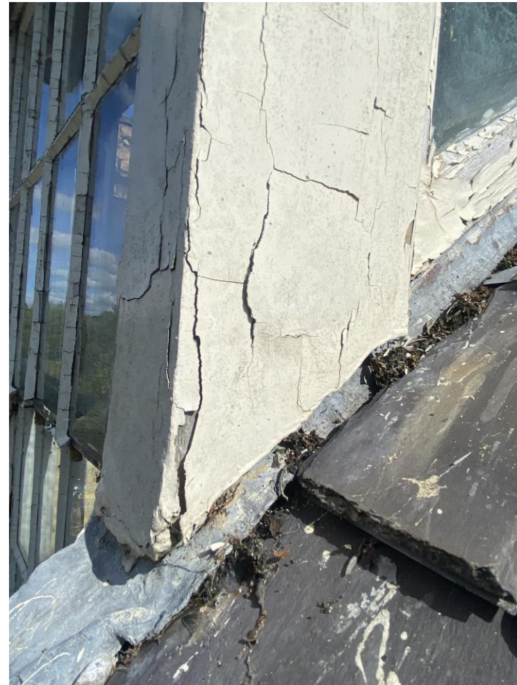
Decay at base of Corner supporting post
