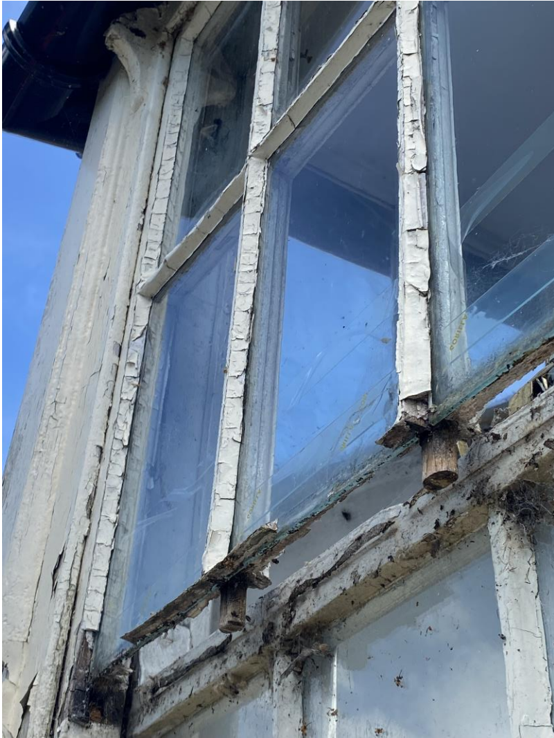
Missing bottom rail of top sash caused by water ingress and wet rot due to poor maintenance and repairs.
