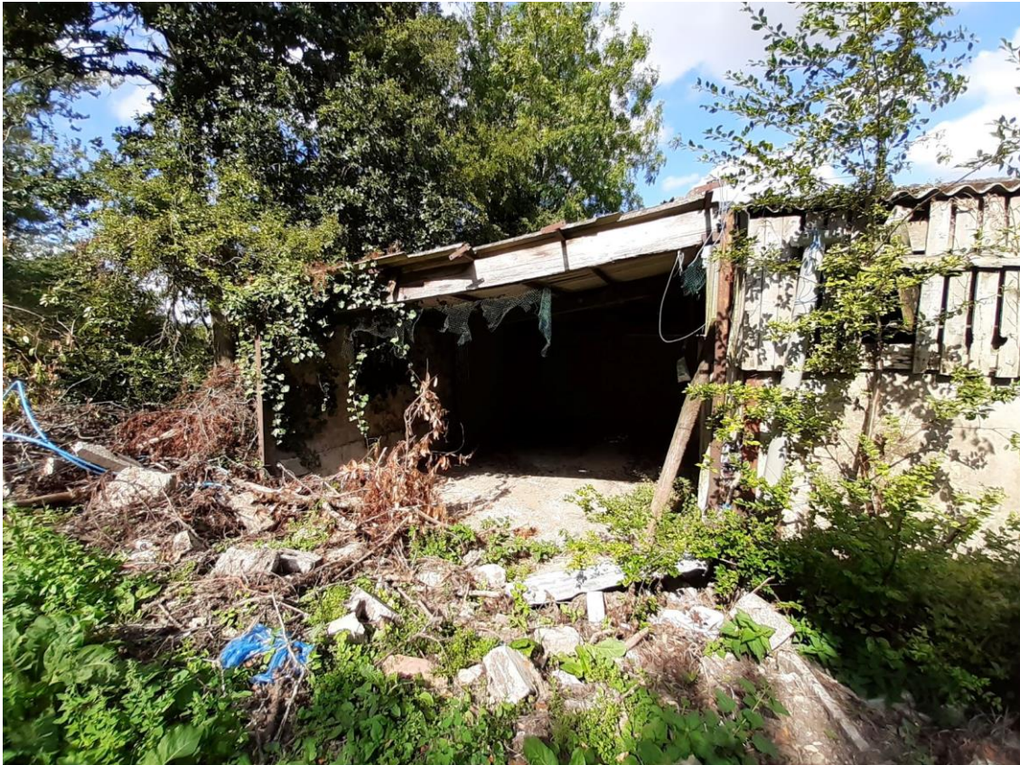
Image 5: Dilapidated lean-to structure to West of barn.
