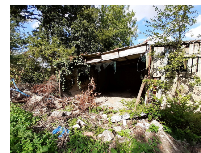
Site Photo 03. Existing South elevation of open barn at rear viewed from bank to side.
