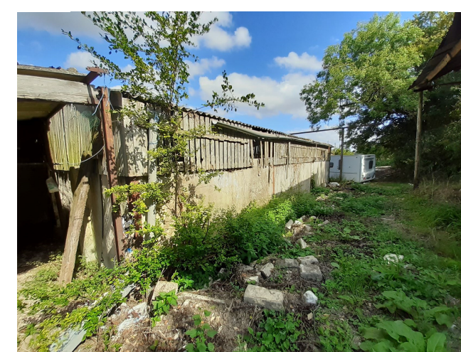
Site Photo 02. Existing South elevation of South Barn viewed from bank to side.
