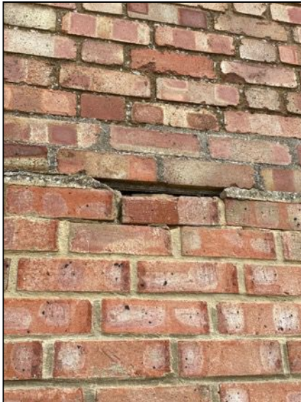
Figure 24 – Gap over the bricked-up window on the south-west elevation of Building 4
