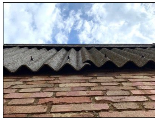
Figure 25 – Gaps under the corrugated asbestos on the south-west gable end of Building 4
