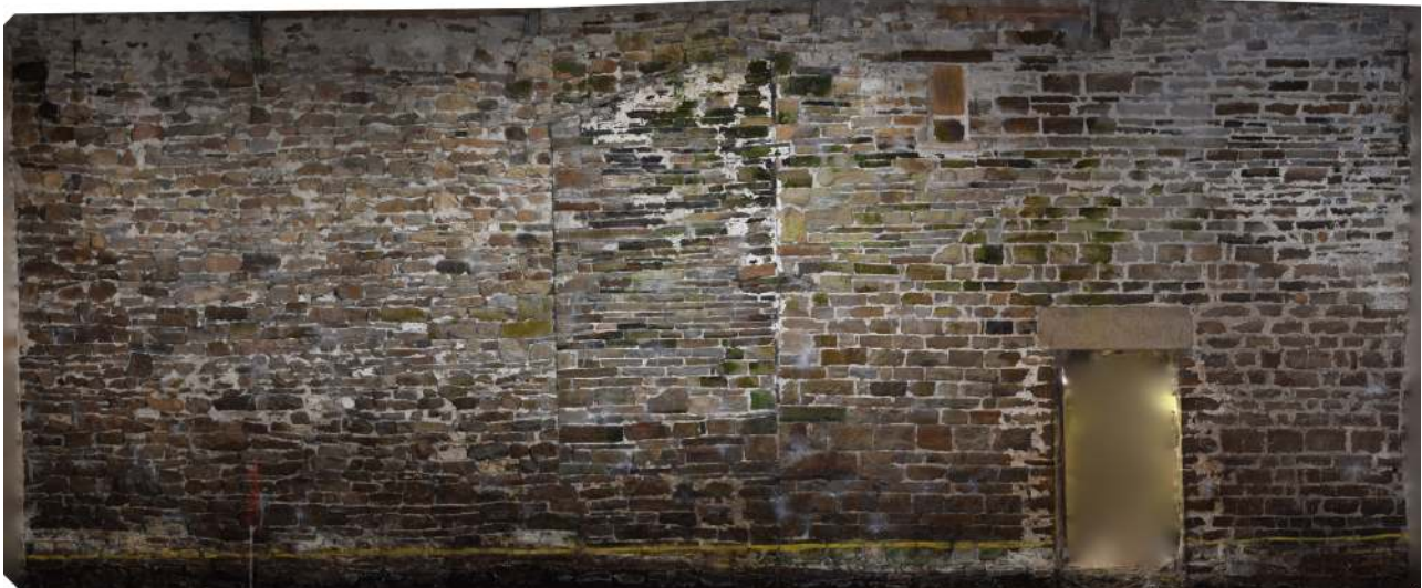
Plate 27. Photogrammetric reconstruction of the internal north-facing wall showing multiple phases of construction
