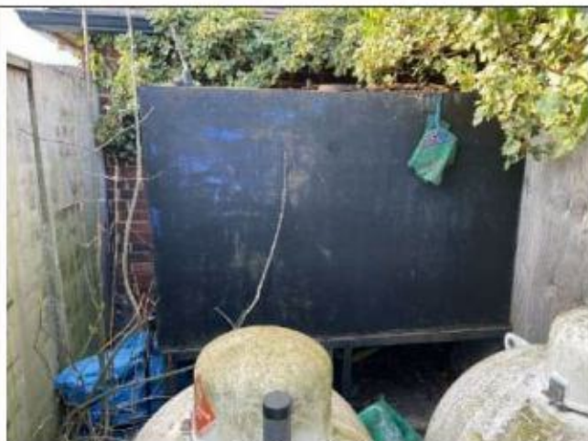
Photograph 14 Above ground LPG tanks and oil tank in residential garden.
