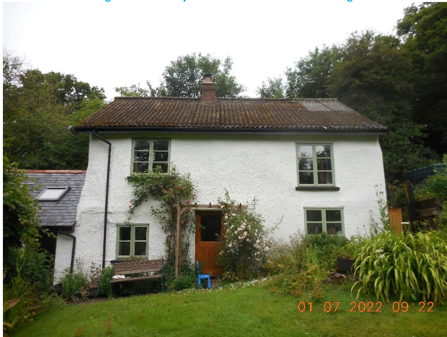
Photo 1: Eastern aspect of cottage showing corrugated sheets
