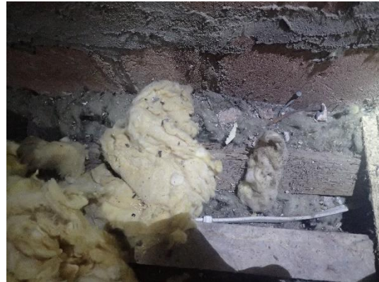
Figure 5. Brown long-eared droppings on insulation next to the north gable wall
