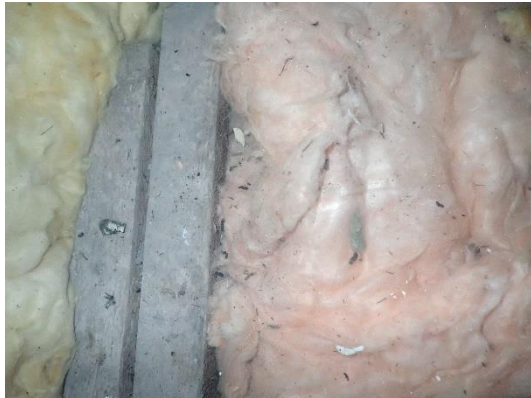
Figure 4. Brown long-eared droppings on insulation next to the chimney
