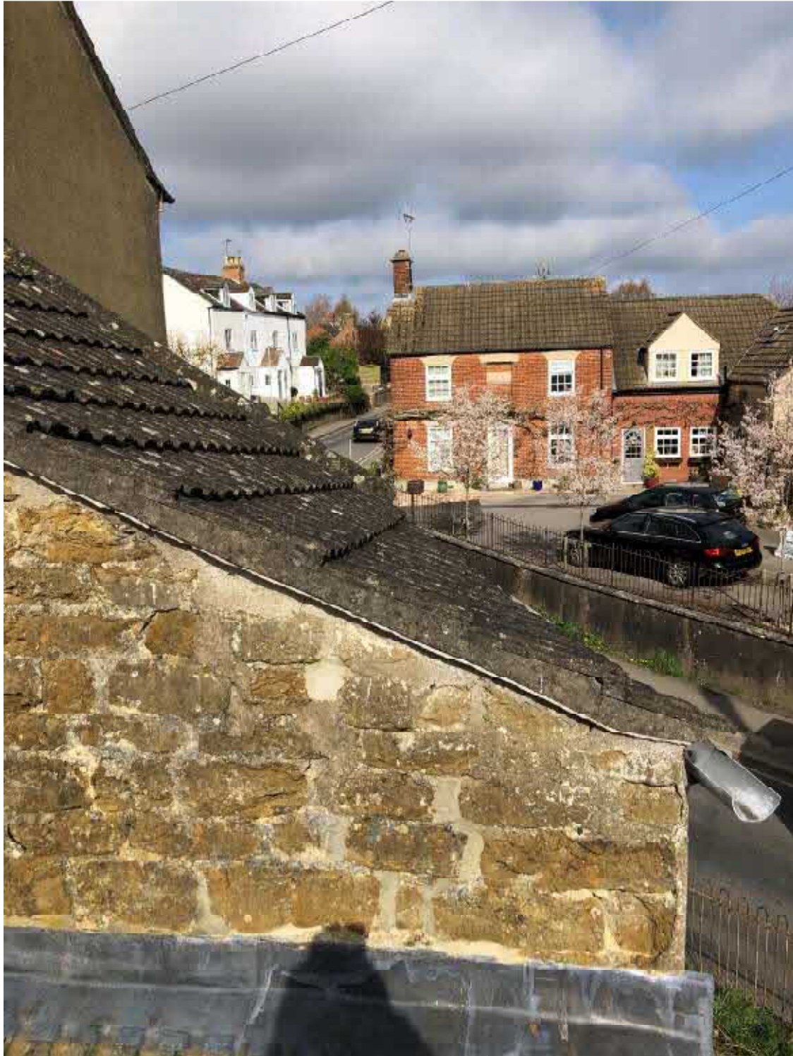
Fig 4: View north across the staircase extension roof looking up Chapel Street showing neighbouring buildings.
