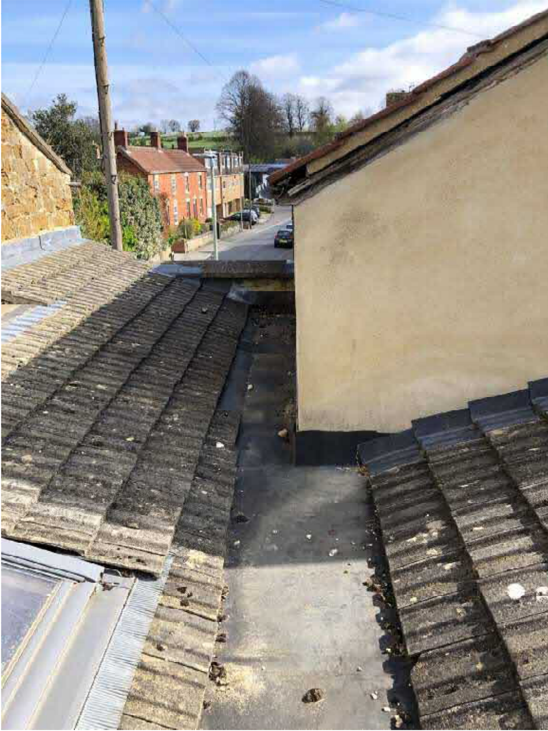
Fig 2: View towards Station Road from the valley between the two roof slopes over the covered area at the back of the house. The rendered building is the annexe.
