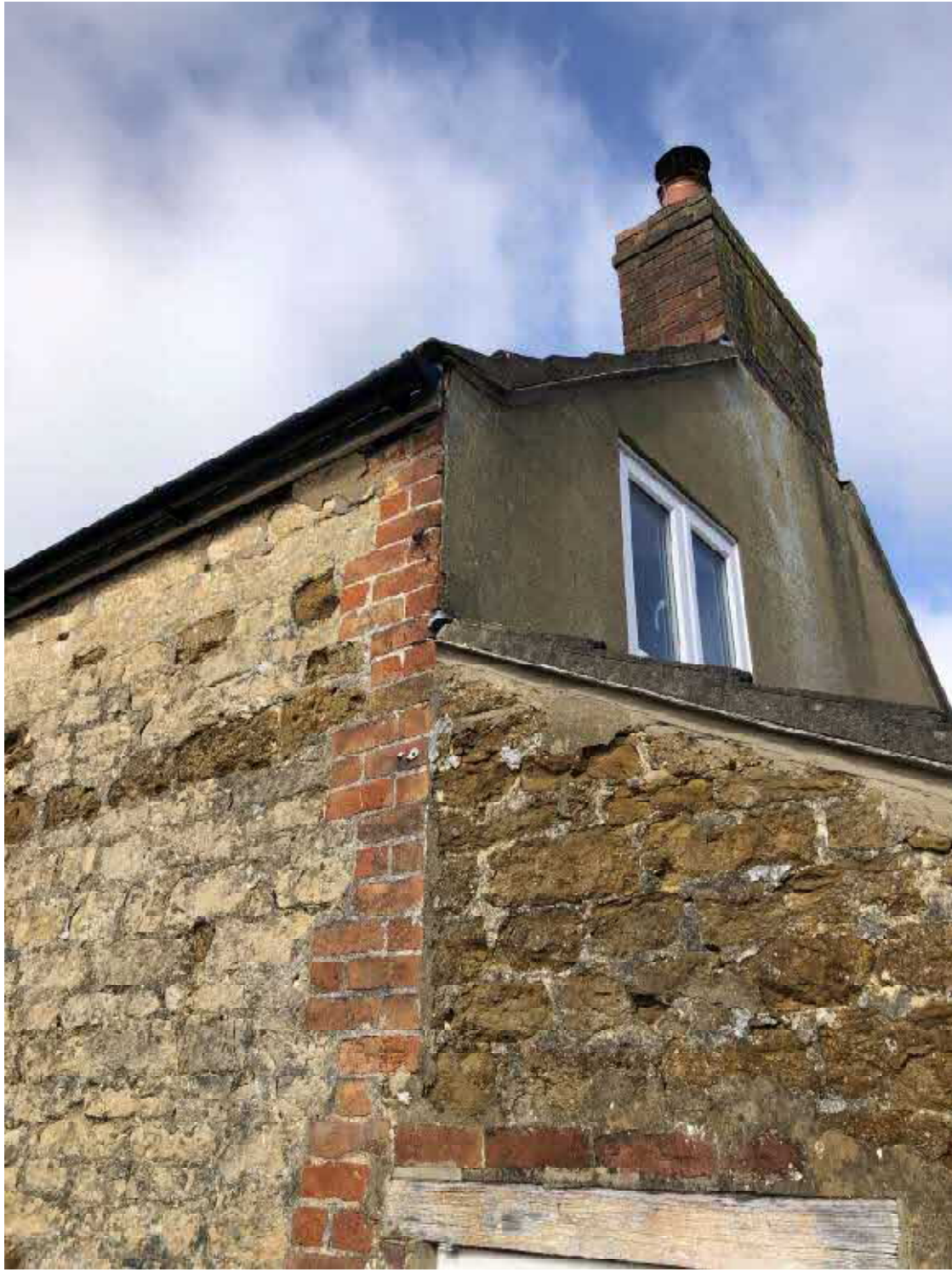
Fig 3: View from the flat roof link showing the staircase extension and the gable end of the main house. A different stone has been used for the staircase extension from that of the rear wall.
