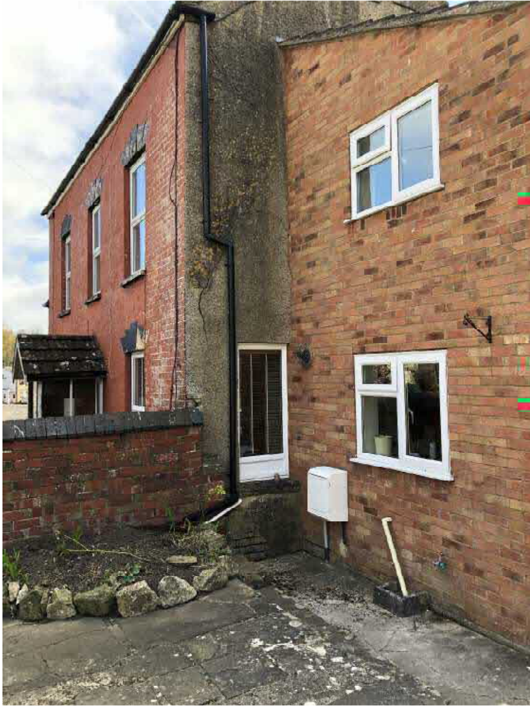
Fig 6: The junction between the modern extension and the main house. The mixture external materials can be seen.
