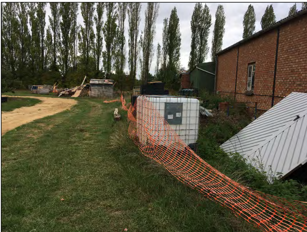
Photograph 14: The area to the rear / west of the buildings, which was covered in grass and in use for the storage of building materials and materials arising from the development of land to the north.
