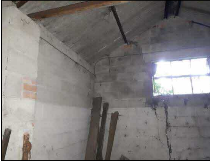
Photograph C5: A records of the interior south-western roof space and window structure at the time of survey.
