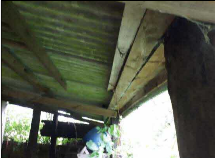
Photograph C1: A potential roost features in the gaps between roof beams of the building (as indicated by a red arrow).
