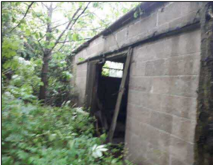
Photograph C4: Broken door of the building allowing free access for birds and bats.
