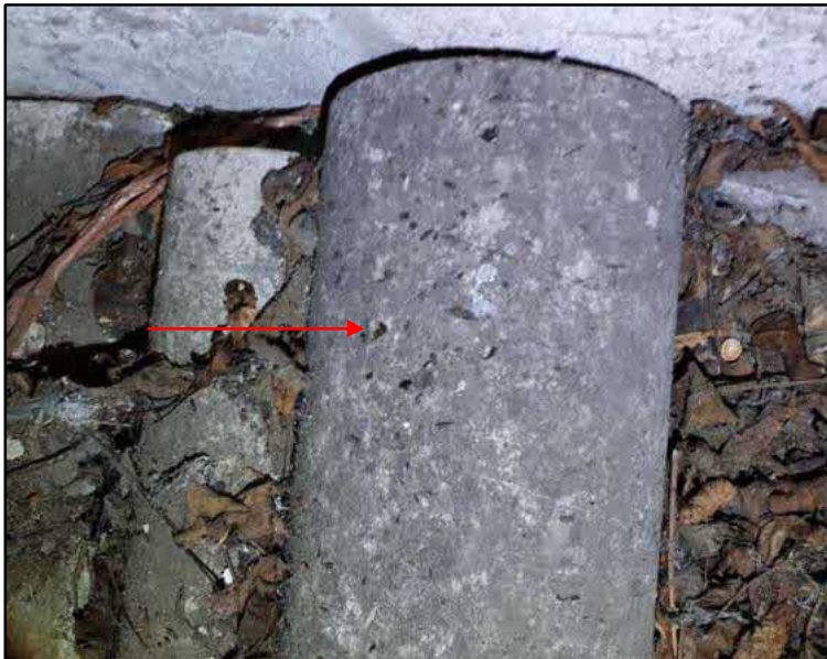
Photograph C13: The bat dropping observed during the internal building inspection in 2019.
