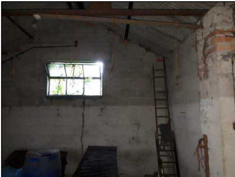
Photograph C9: A record of the interior north-eastern roof space and window structure at the time of survey.
