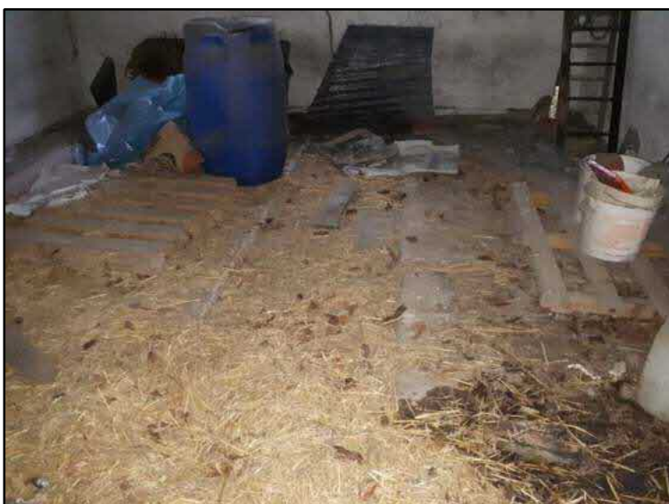
Photograph C10: A record of the interior north-eastern floor structure of the building at the time of survey.
