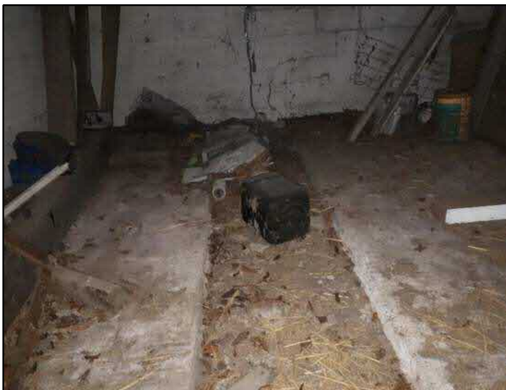
Photograph C7: A record of the interior south-western floor structure of the building at the time of survey.
