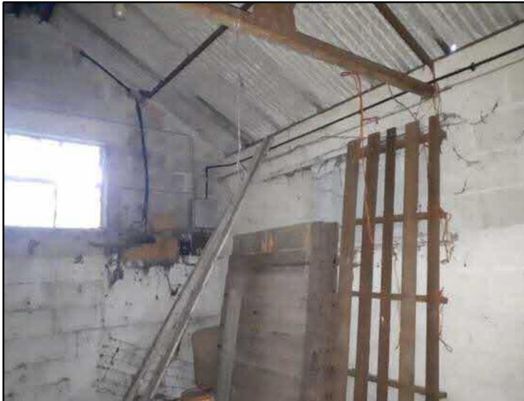
Photograph C6: A record of the interior south-western roof space and window structure at the time of survey.
