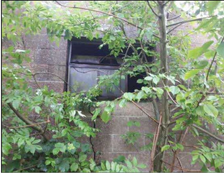
Photograph C3: Broken windows of the building allowing free access for birds and bats.
