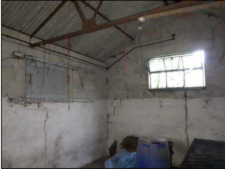
Photograph C8: A record of the interior north-eastern roof space and window structure at the time of survey.
