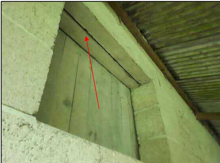
Photograph C2: A potential roost feature in the gap between brick work in a covered window of the building (as indicated by a red arrow).
